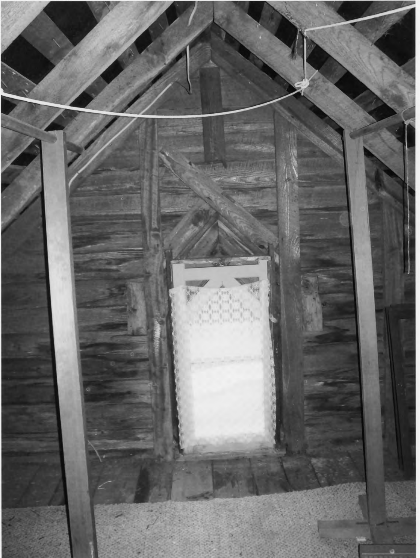
Tunnell - West House_Sussex County_DE attic construction detail (main block of house) showing lancet window framing (south gable end) and roof rafters
