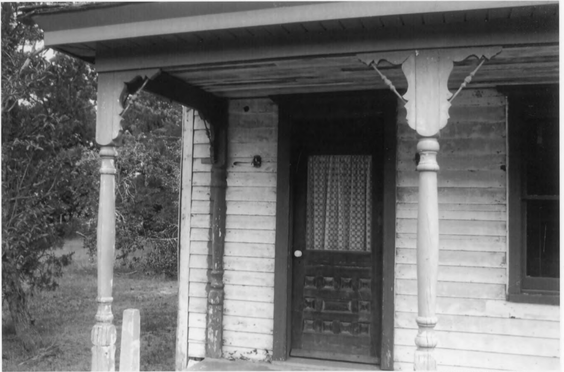
Tunnell - West House_Sussex County_DE original glass and decorative paneled front door (west facade)
