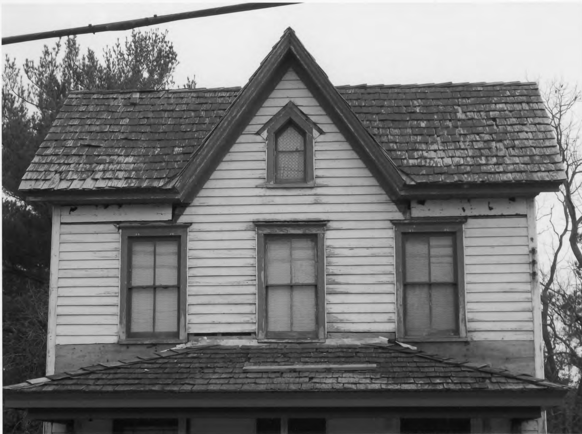
Tunnell - West House_Sussex County_DE west facade detail - second floor features original clapboards, windows, roof cornice with plain frieze (where decorative brackets may have been nailed)
