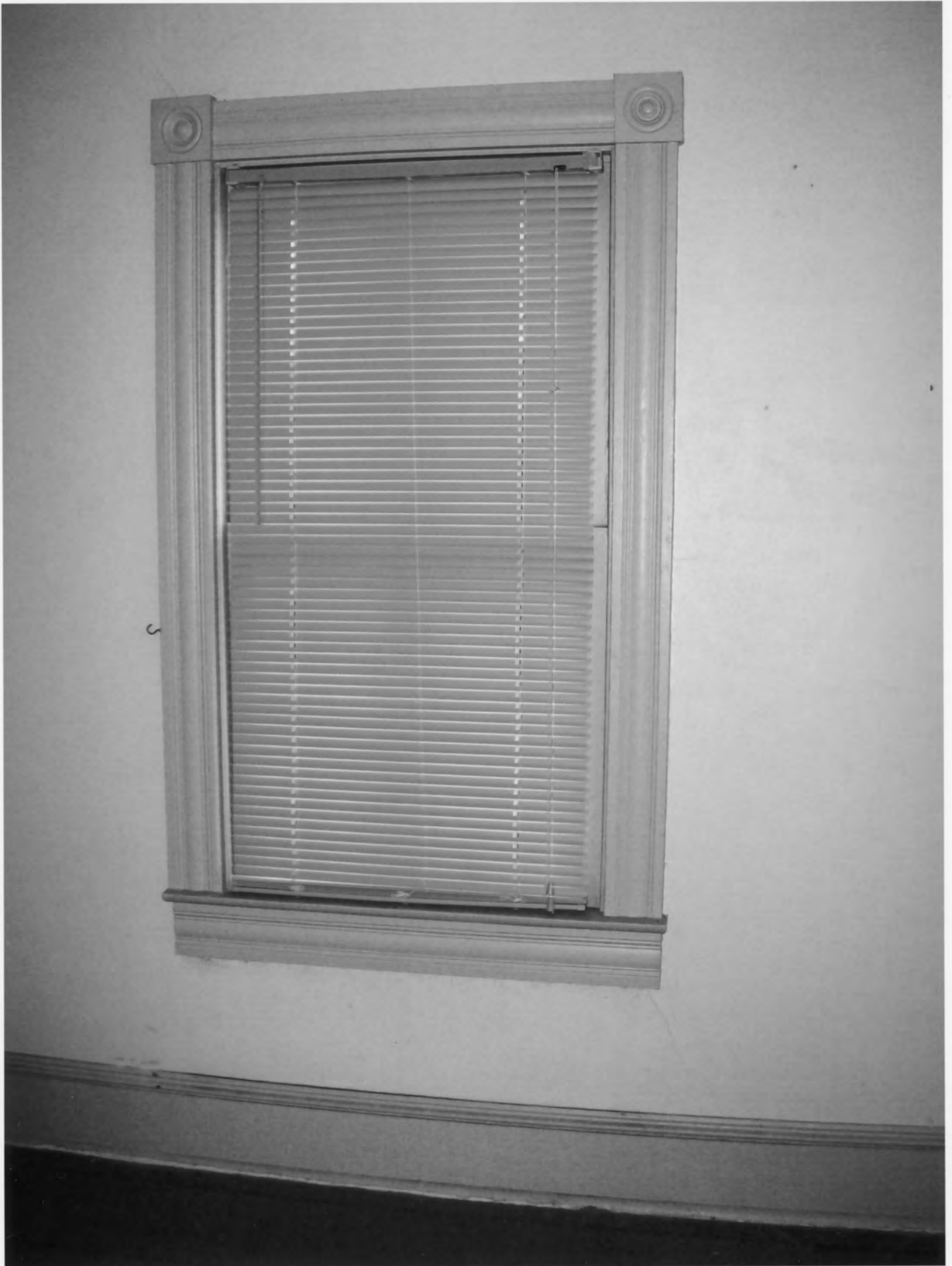
Tunnell - West House_Sussex County_DE original second floor window with moulded trim casing and sills, decorative bulls-eye corner blocks, and baseboards 20 of 25
