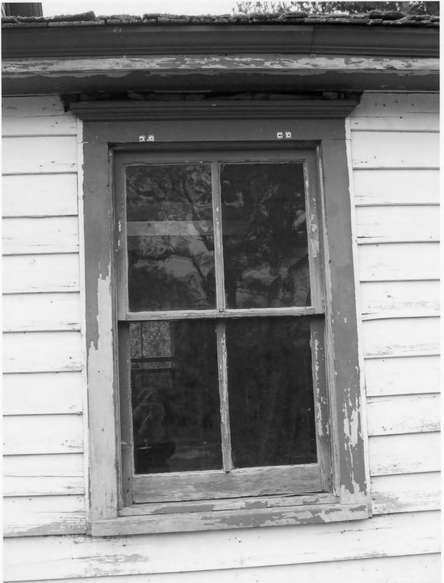
Tunnell - West House_Sussex County_DE detail of original c. 1900 window (south elevation, first story wrap around addition)
