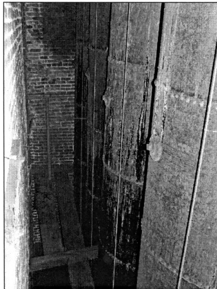
Figure 26: base of iron tanks, view west from entrance door (photo by Jim Jacobsen, May 2007)
