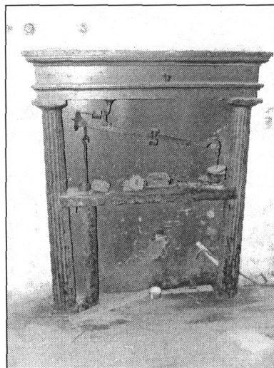
Figure 28: Scale in wall on ground floor of main building, view northeast (photo by J. Jacobsen, July 2007)
