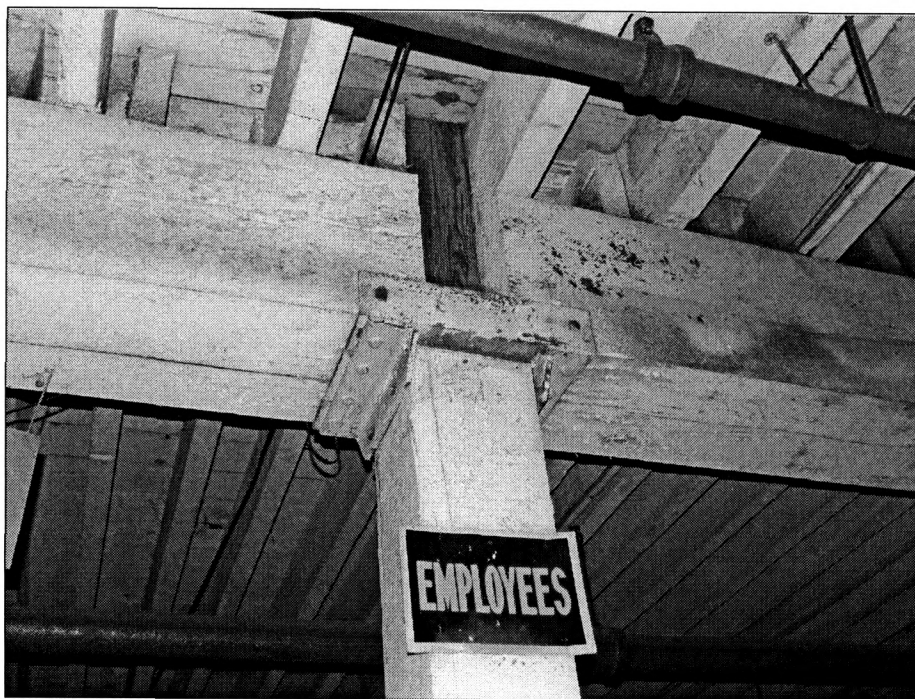
Figure 19: Column/beam transition from first floor to second floor column in courtyard area and simple metal collar, view northwest (photo by J. Jacobsen, May 2007)
