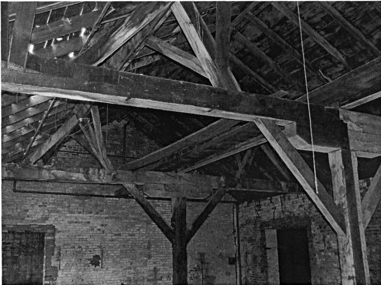
Figure 22: Roof framing, east room, south wing, view northwest (photo by J. Jacobsen, May 2007)
