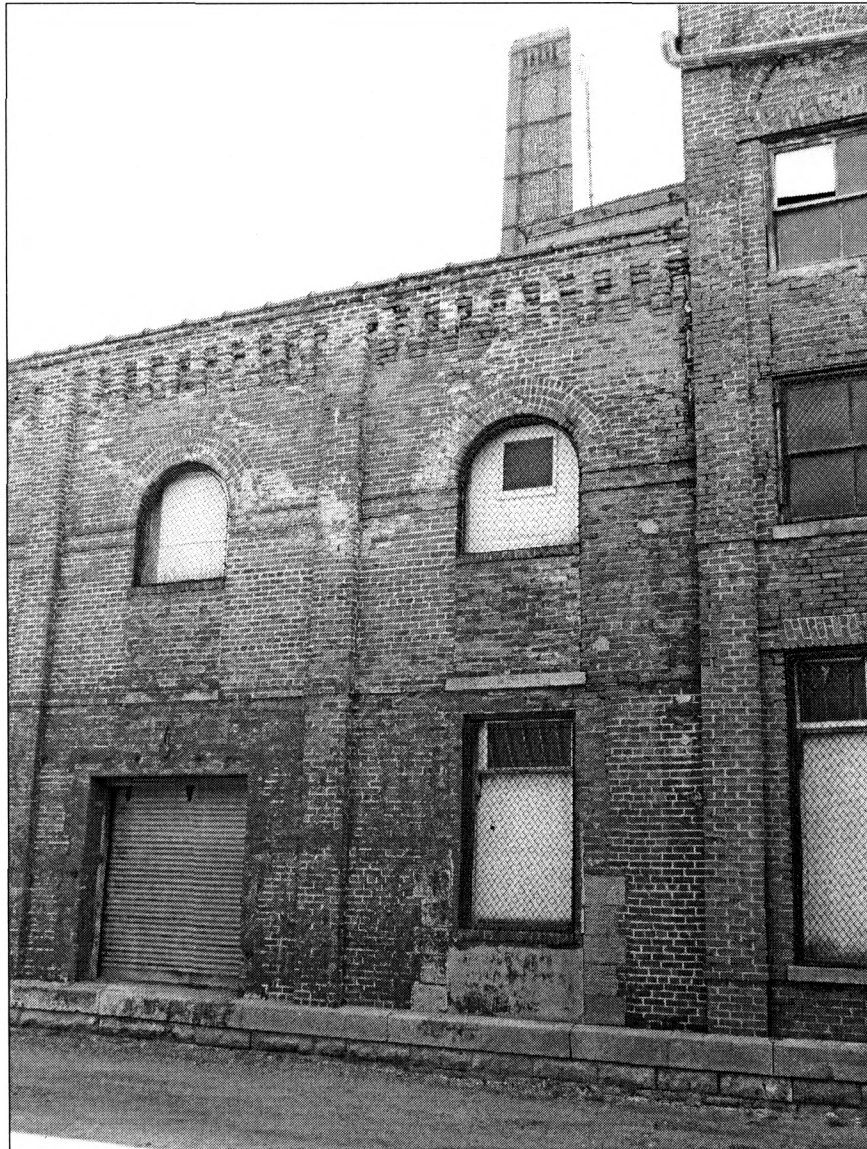
Figure 11: Engine and boiler house, north wall, view southeast (photo by J. Jacobsen, May 2007)
