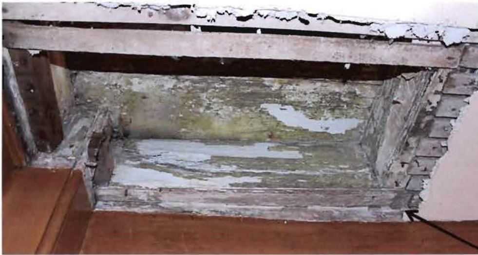
Figure 10: southeast corner of the kitchen with some of the ceiling removed to show an original beaded joist (heavily painted) to the right and the wrapped corner post to the left. The arrow points to a peg in the girt that secures the tenon on the joist. View south.
