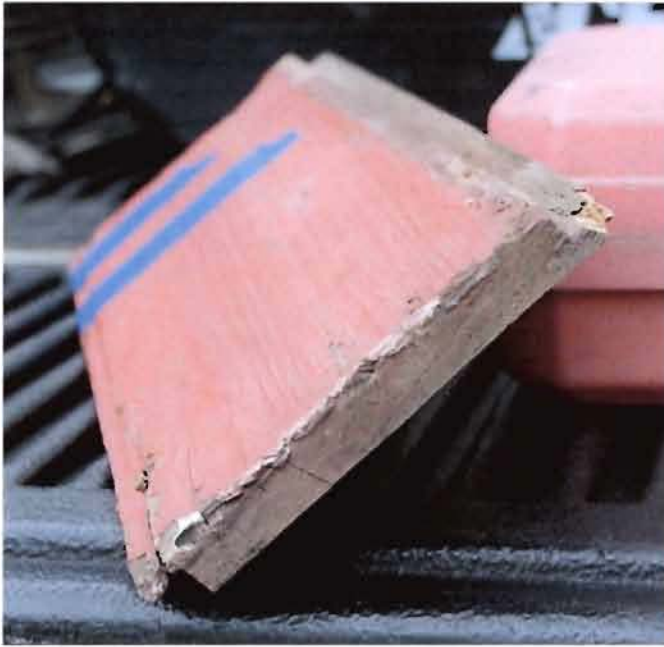
Figure 7: piece of original ship lap siding with a rabbeted top edge and a beaded + rabbeted bottom edge.
