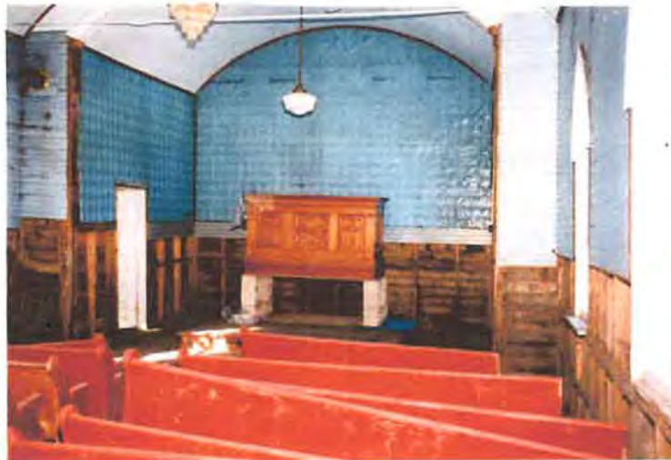
Fig. 19: Photo of structure during interior restoration, ca. 2002 (courtesy of Fort Pembina Historical Society)
