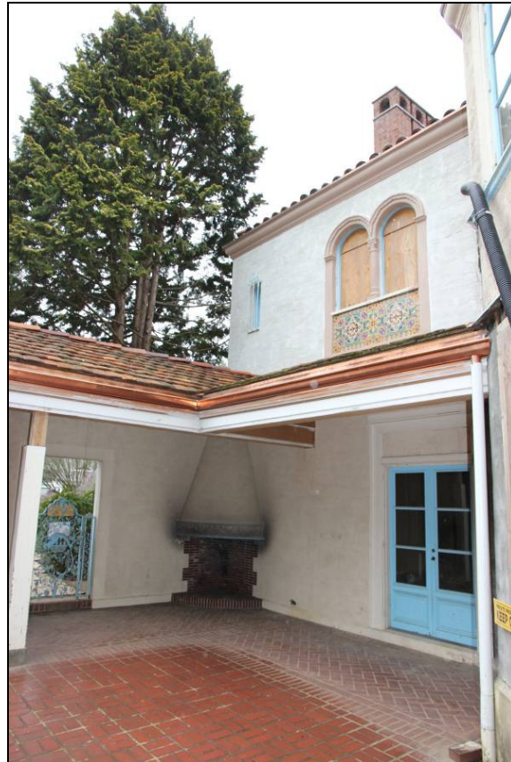
Photo 6 of 32: West elevation showing French doors from Living Room, faience tile panel under upper windows, and outdoor fireplace.
