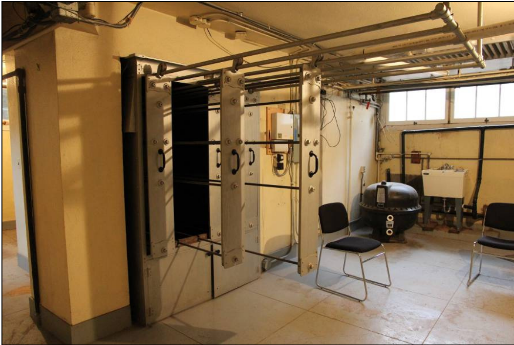
Photo 31 of 32: Commercial dryer located in the laundry area in the basement.
