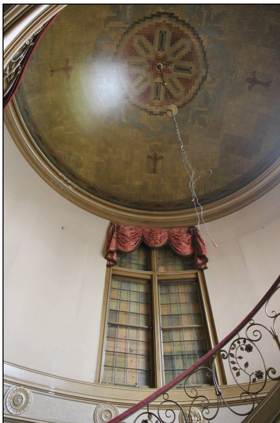
Photo 12 of 32: Stair Hall dome with tinted leaded glass window and faux mosaic painting (chandelier was in storage at time of photo).
