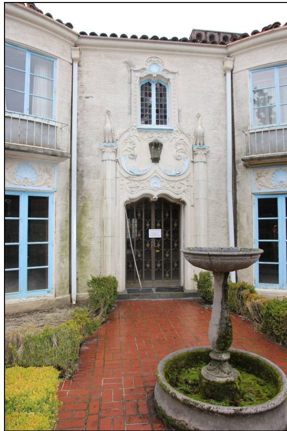
Photo 4 of 32: South entry from terrace, showing doors, leaded-glass window & elaborate cast surround.
