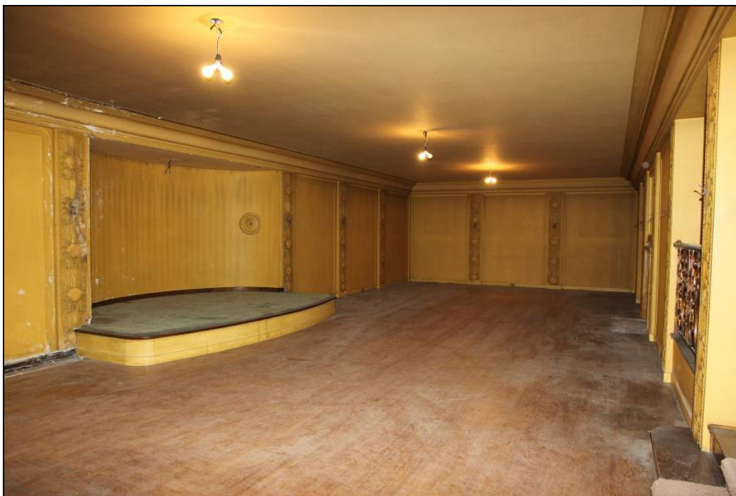
Photo 30 of 32: Ball Room showing built-in stage on south wall (light fixtures in storage at time of photo).
