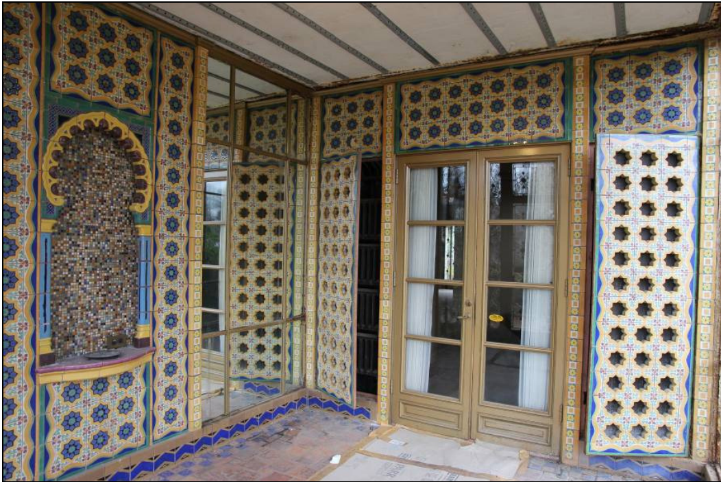
Photo 10 of 32: Entry porch interior – south and east walls – showing tile work, main entry doors and mechanical alcoves flanking doors.
