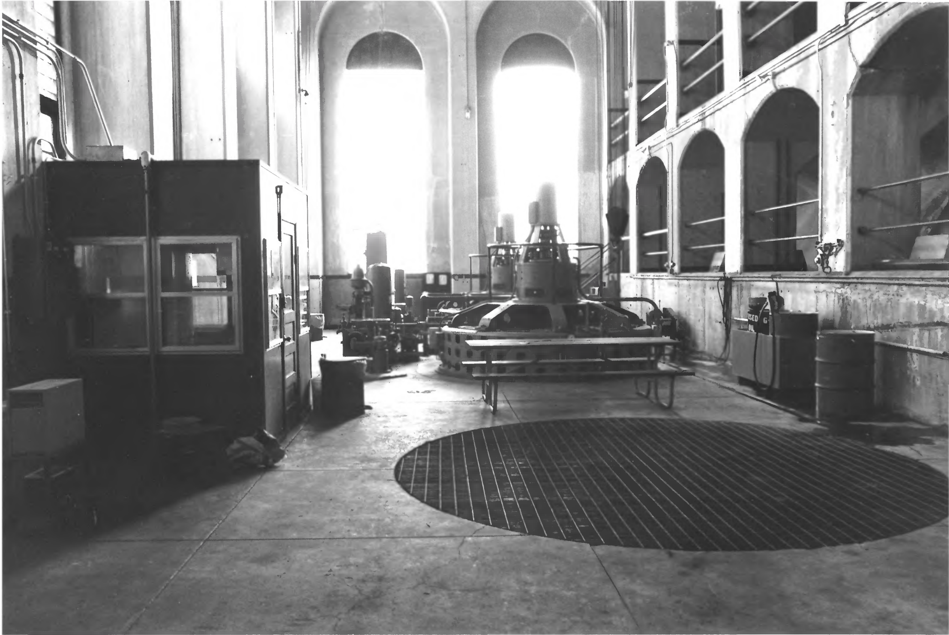
Lake Umbagog Hydroelectric Generating Plant Mazeppa Twp., vicinity of Mazeppa, Wabasha Co., MN 010526-12
