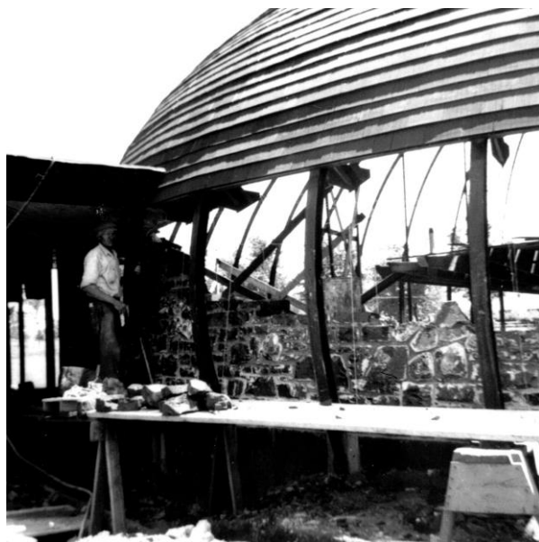
Photograph of construction of coal and glass masonry wall adjacent to northeast bathroom June 1950.
