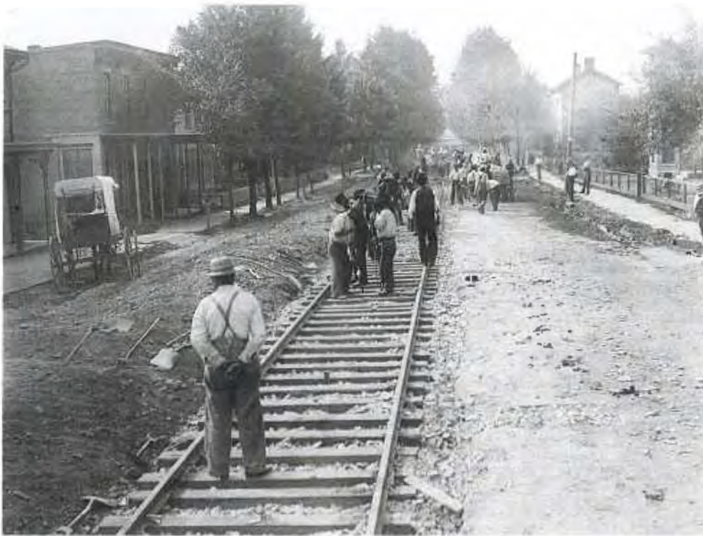
Figure 2: Interurban Railway tracks being laid on South State Street, looking south from College Avenue, 1895
