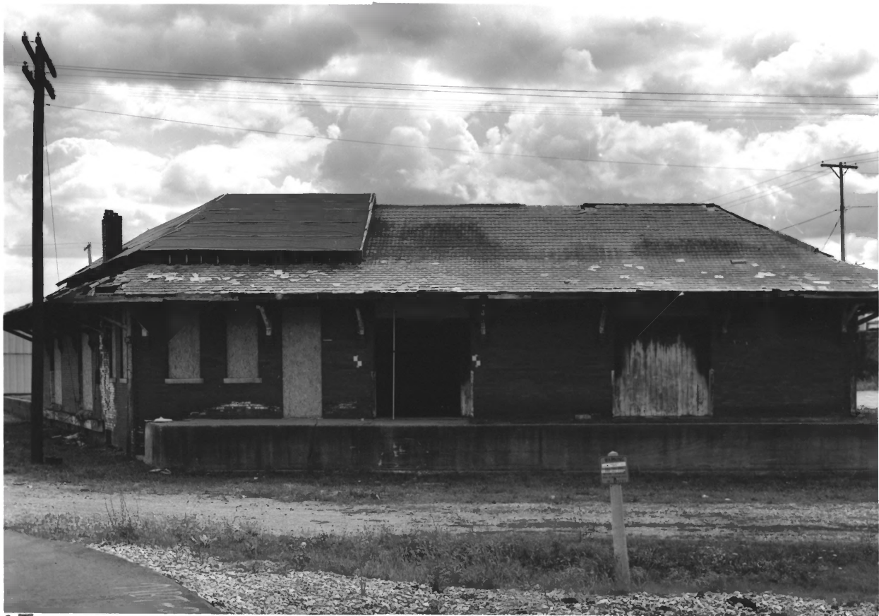
C. & E. I. FREIGHT DEPOT, 42 S. WATER ST., CLINTON DOWNTOWN HIST. DIST., VERMILION CO., IN, PHOTO No. 7
