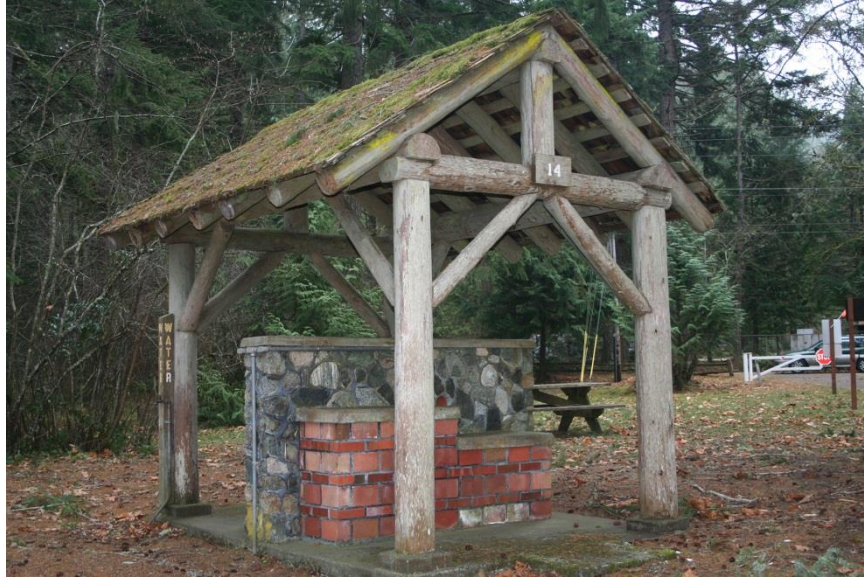
0009: Building 14, small kitchen, one of three, west and north elevations, looking southeast.
