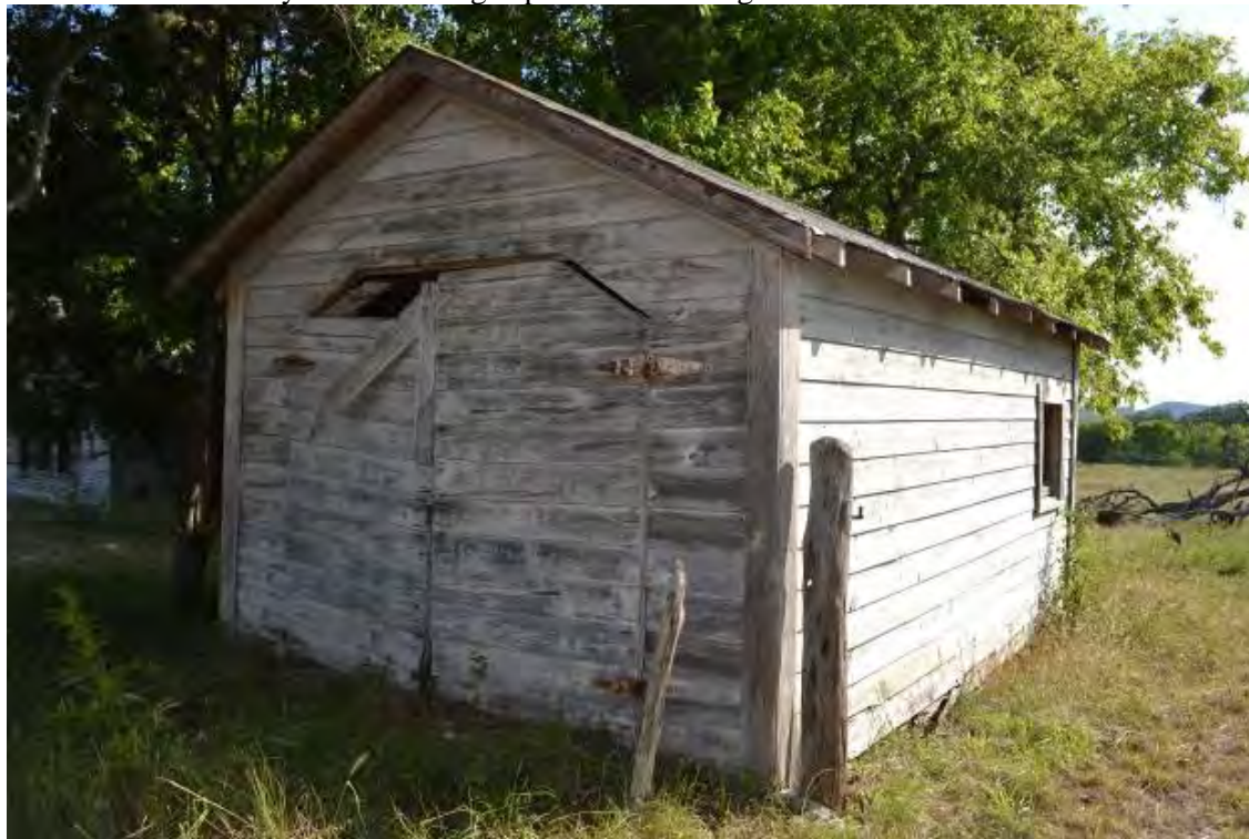
Photo 13 – Garage east and north elevations, camera facing southwest. The garage stored a vehicle, and the western end contained a utility room with a gas-powered washing machine.
