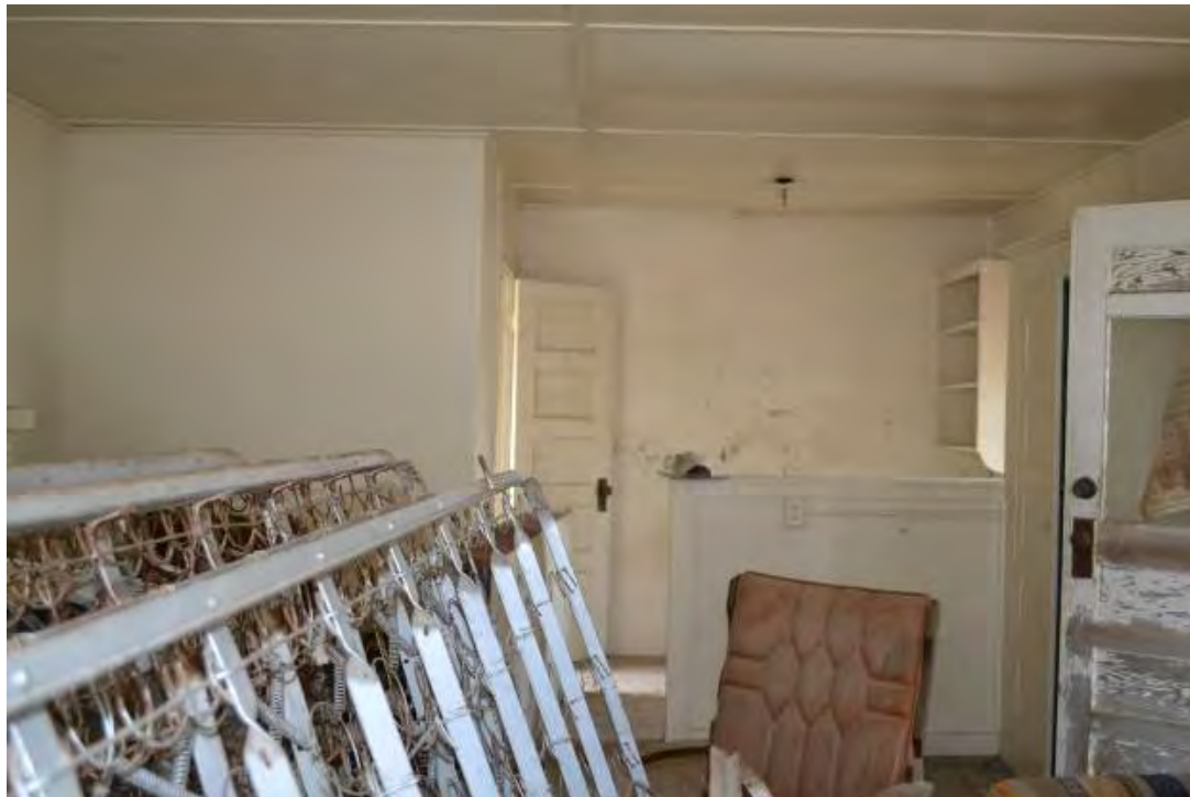
Photo 21 – Cabin #5 interior, camera facing north. Most cottages featured a kitchenette, shown here behind the half-wall.
