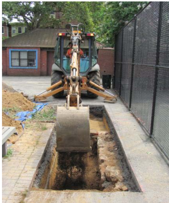
Figure 26: Archeologists backfilling a trench after 2013 investigation was completed (adjacent fence is along tennis court; building in rear is Recreation Building). The southern portion of the tennis court, and the entire Recreation Building, are over the burial ground site.
