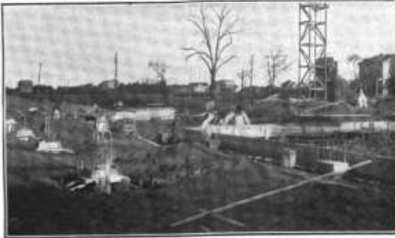
The Piers at Ground Level. The Forms for the Footing Walls in Place.
