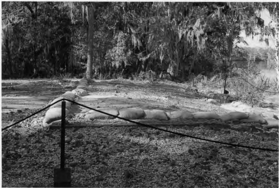
89. Foundation of the Garden House, facing north Drayton Hall 3380 Ashley River Road Charleston County, South Carolina Photograph by Lissa Felzer, 12/10/2007
