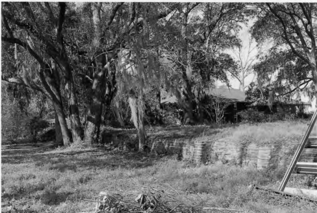
69. Retaining Walls/Foundation Walls, facing south Lambs Phosphate Mining Facility Lambs Road Dorchester County, South Carolina Photograph by Lissa Felzer, 3/8/2008
