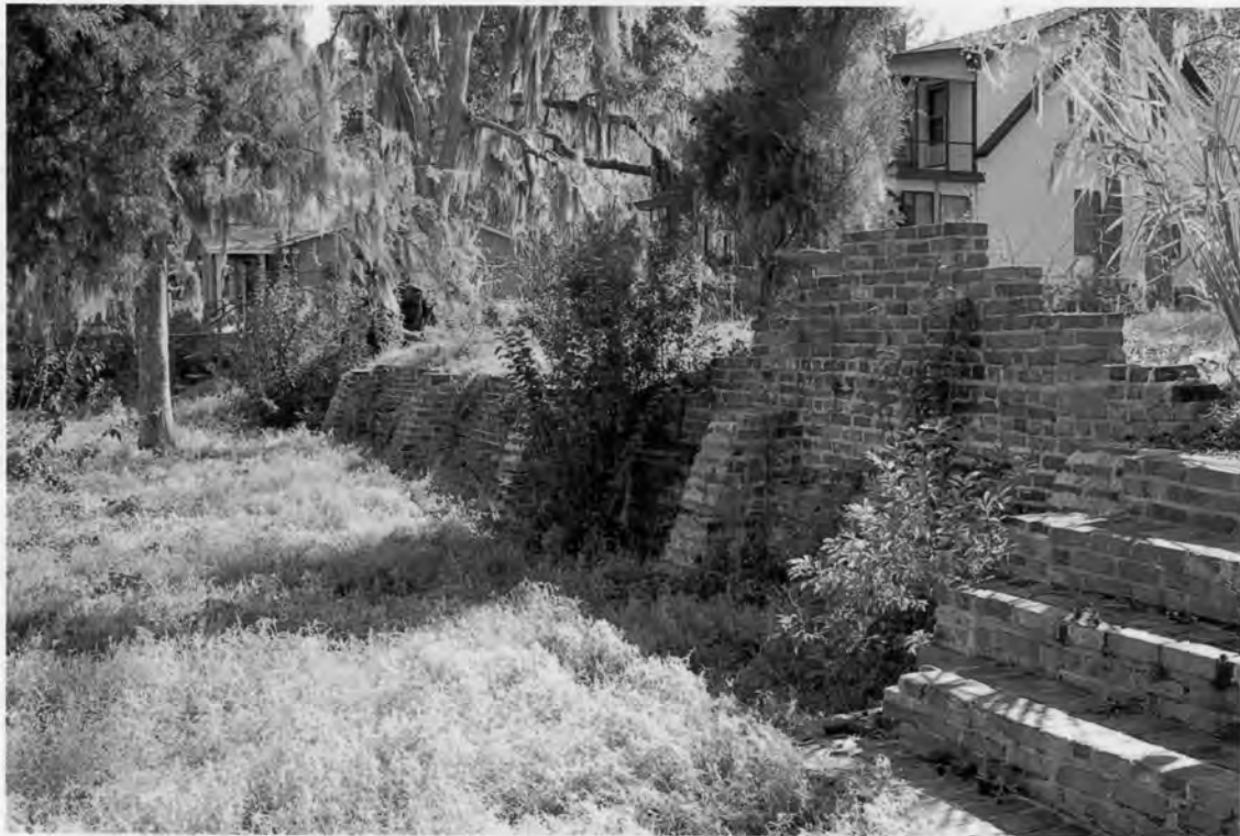
70. Retaining Walls/Foundation Walls, facing north Lambs Phosphate Mining Facility Lambs Road Dorchester County, South Carolina Photograph by Lissa Felzer, 3/8/2008
