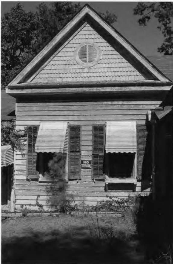
61. Club House, partial south elevation Millbrook Plantation Ashley River Road Charleston County, South Carolina Photograph by Lissa Felzer, 3/2/2008
