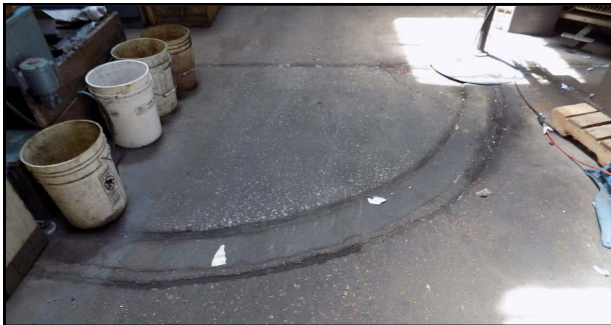
Figure 15: Interior evidence of location of 1920s equipment installations; there are two identical details still extant in the rear warehouse floor. Source: Matt Bivens, 6-2016.
