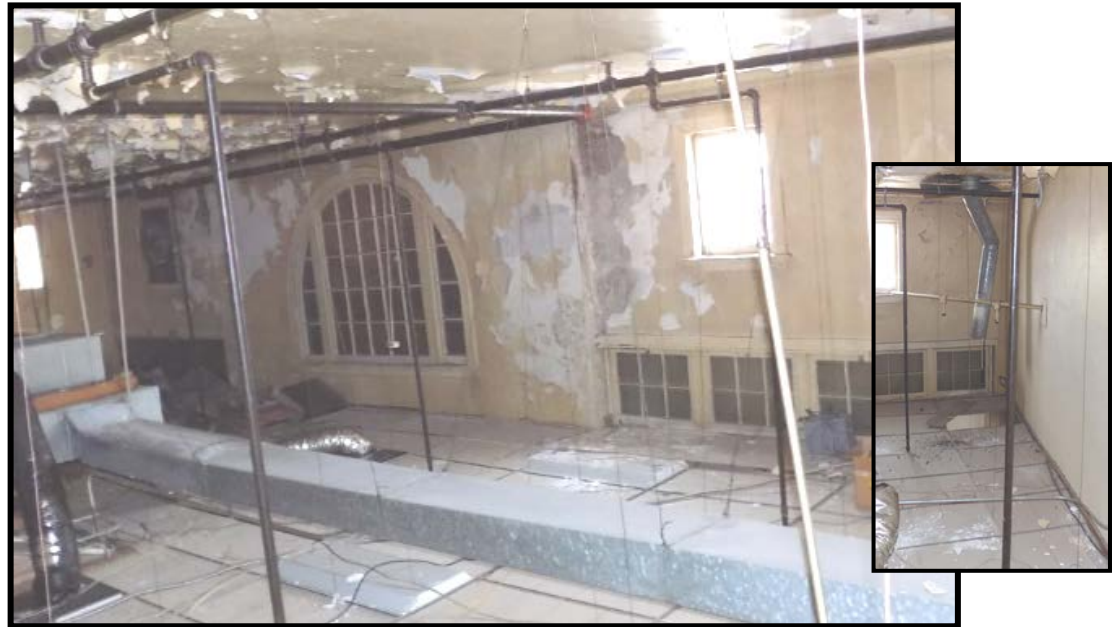
Figure 1: Interior side of front windows covered by boards. Original fabric is intact. Source: Matt Bivens, 6-2016.
