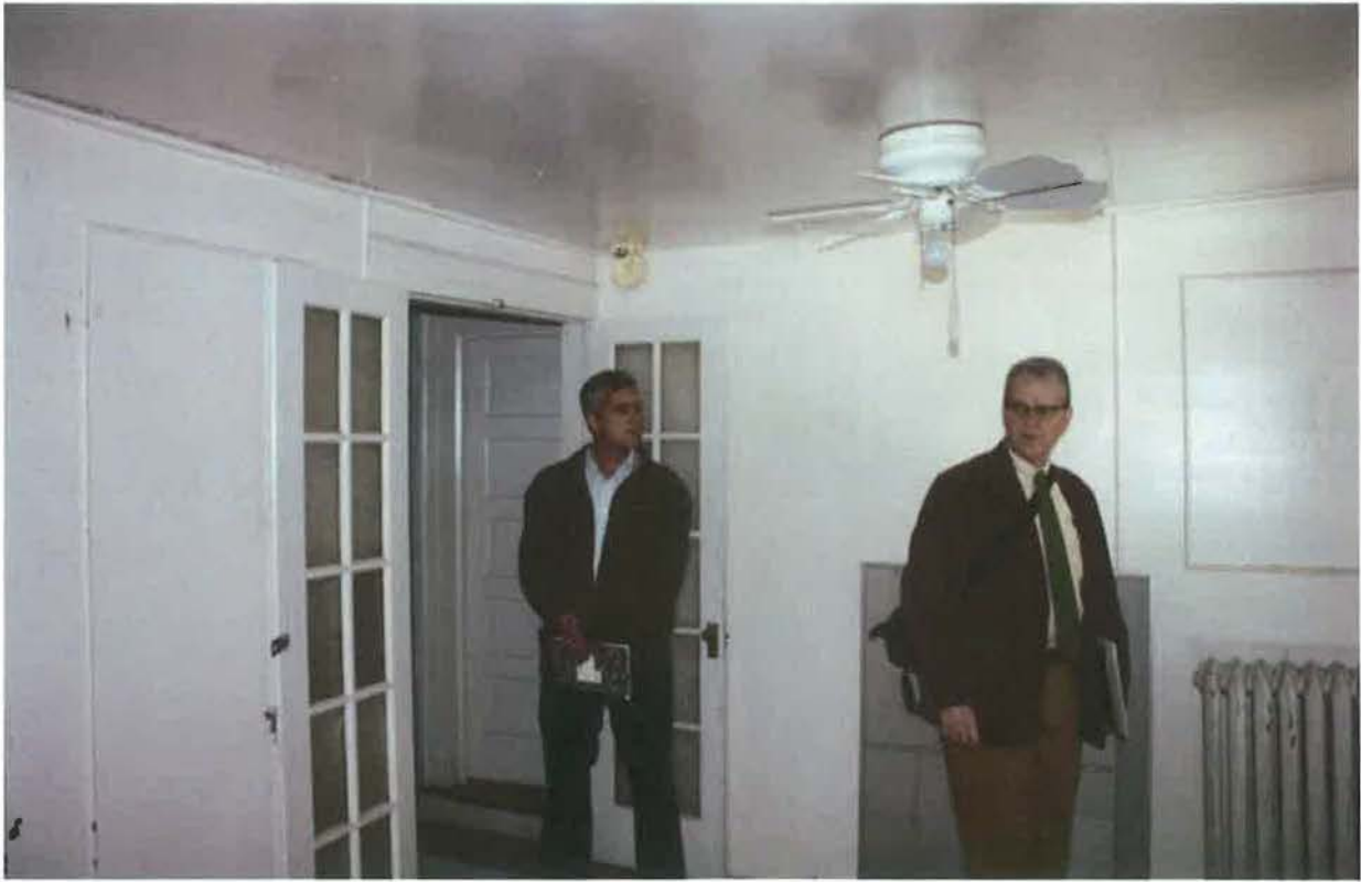
Rear addition off of the stair landing between first and second floors
