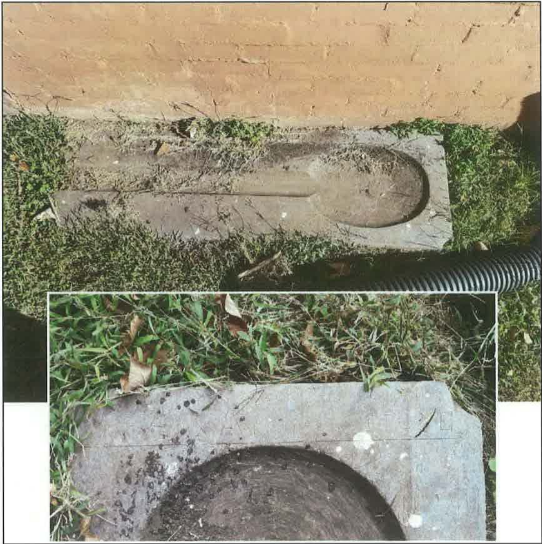
Figure 21: Carved soapstone splash guard, with detail, at the southeast corner of Wyndhurst.
