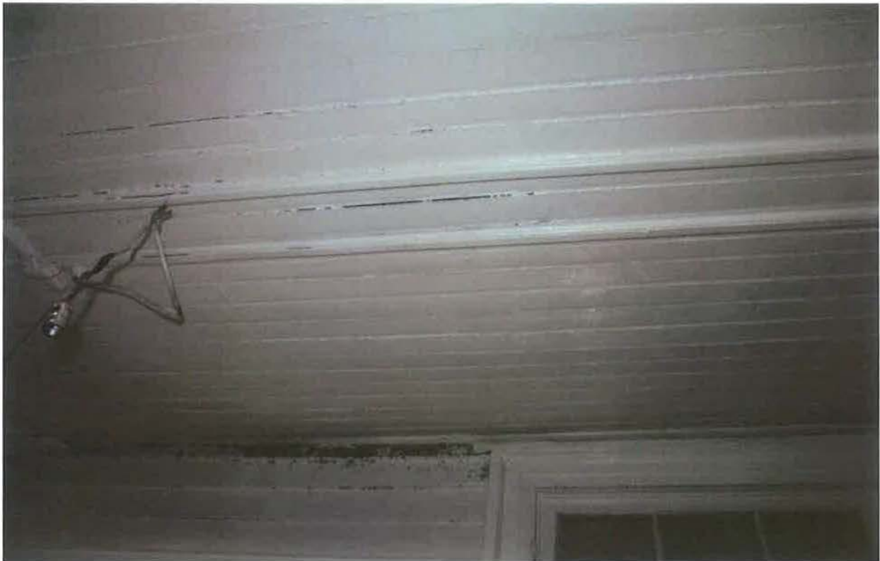
First Floor, rear NE addition adjoining main house, beaded board ceiling detail
