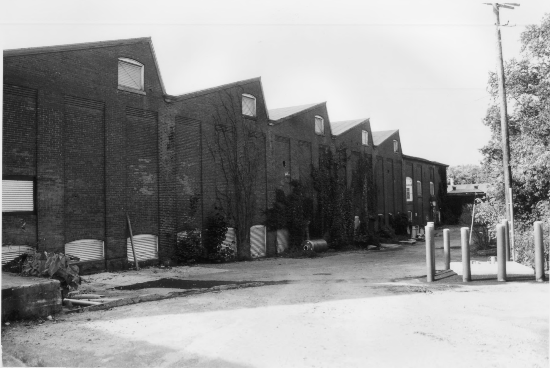
Dye House with Weave Shed at East Greystone Mill Historic District North Washington, Washington County, Maryland Photograph Number 4
