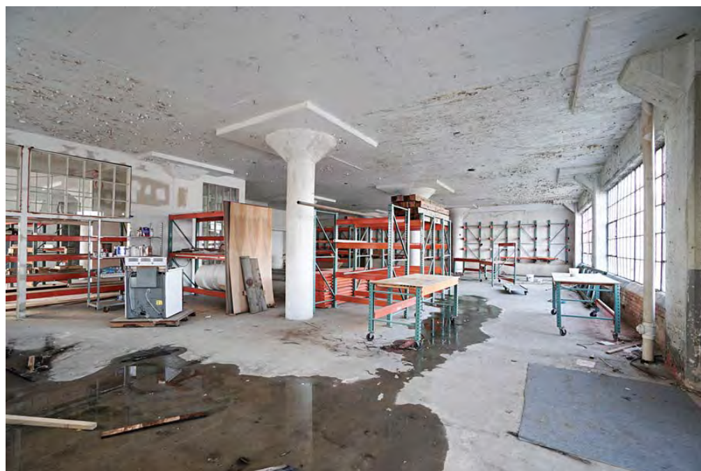
Figure 21: The first floor of the north unit, looking northwest (c. 1930s) and looking west (2017). Partitions, as seen in the bottom image, reflect the original location within the interior space.
