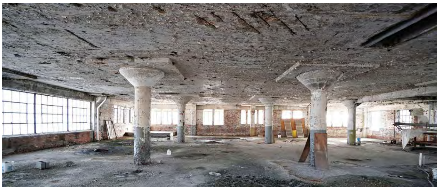
Figure 20: The second floor of the north unit, looking east, c. 1930s (above) and 2017 (below). Note the historic, character-defining features of the interior space vital to the significance of the property, are extant. Key interior materials and arrangement of space as originally designed and constructed, remain.
