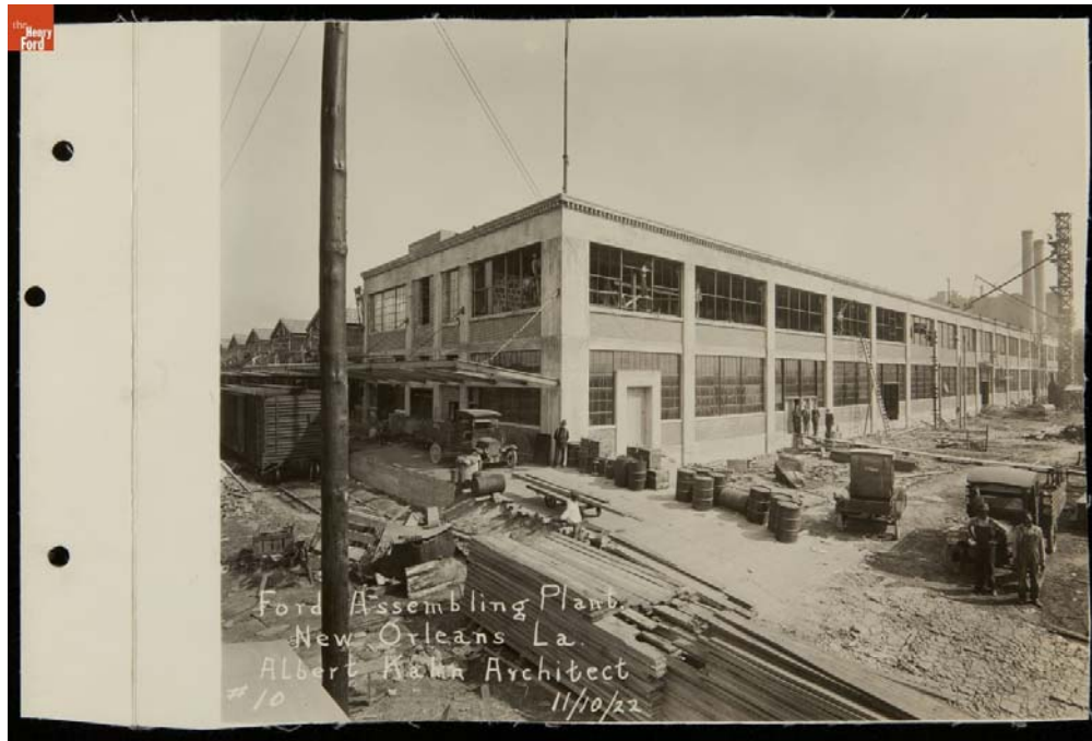
Figure 3. The Arabi assembly plant under construction in November 1922. The Domino Sugar Refinery is visible in the distance. From the Collections of The Henry Ford. Gift of Ford Motor Company.
