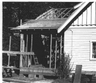
1912 photograph of the Dining Hall's northeast kitchen expansion under construction. Source: Digital copy provided by Carmen Scott.
