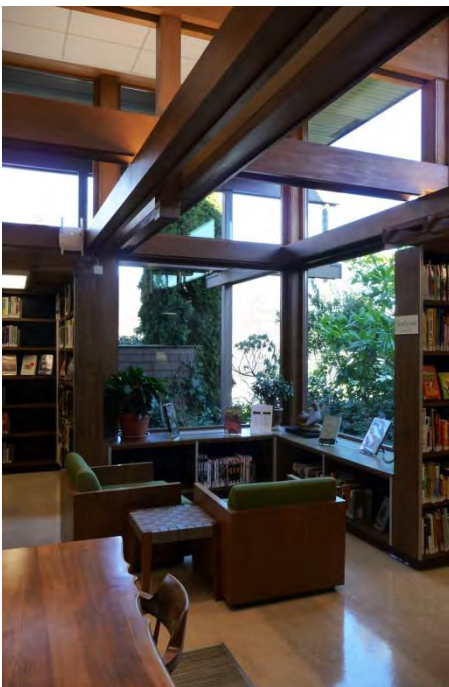
Photo #11 Interior view of northeast corner of reading room and roof overhang, camera facing northeast Photographer: Susan Boyle, January 14, 2015
