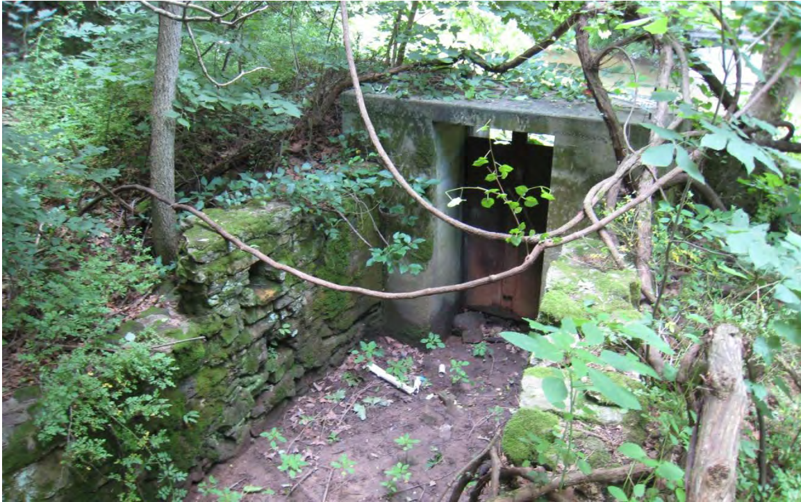
Photograph 1. View of a post-Continental Powder Mill sluice gate at the dam. Note the pockets in the stonework, which likely relate to the superstructure of an earlier gate.
