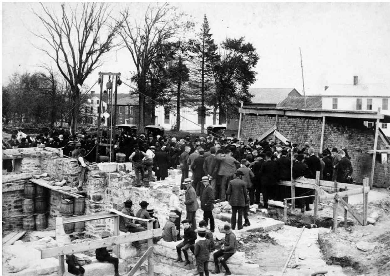
Figure 8.17: Laying the cornerstone of the Conant Memorial Congregational Church, 1890. Note, in the background (l. to r.), the Phinehas Bemis House, Phinehas Bemis Store, Methodist Church, the Black Tavern Barn and Annex, and the Black Tavern (without its front porch). From the Dudley Historical Society collection at Pearl Crawford Public Library; used with permission.
