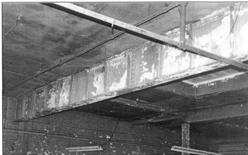
Figure 9: Structural truss above showroom area on second floor, view southeast (Photo by J. Jacobsen, August 2006)
