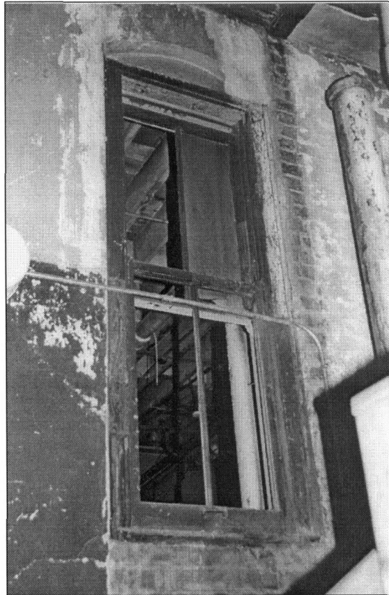
Figure 8: Surviving elongated 2/2 window on former or original rear wall, view northeast (Photo by J. Jacobsen, August 2006)
