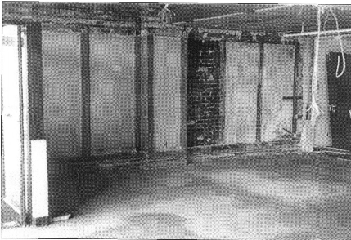
Figure 6: Surviving framed plaster wall panels, east sidewall, surviving tile floor, view southeast (Photo by J. Jacobsen, August 2006)
