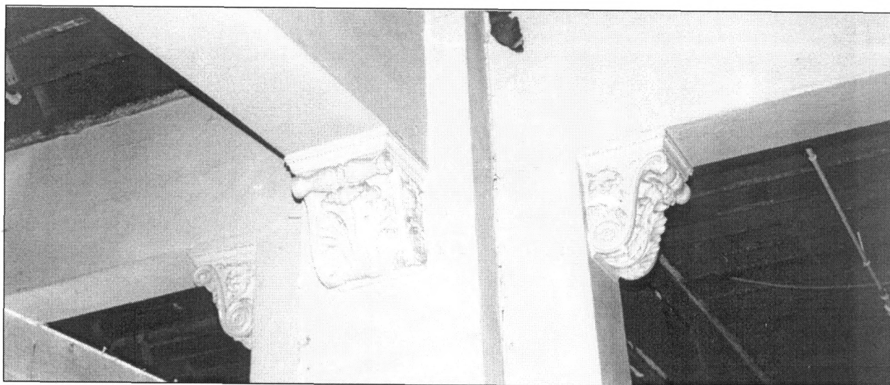
Figure 7: Decorative brackets at showroom juncture of former partition, view southwest (Photo by J. Jacobsen, August 2006)
