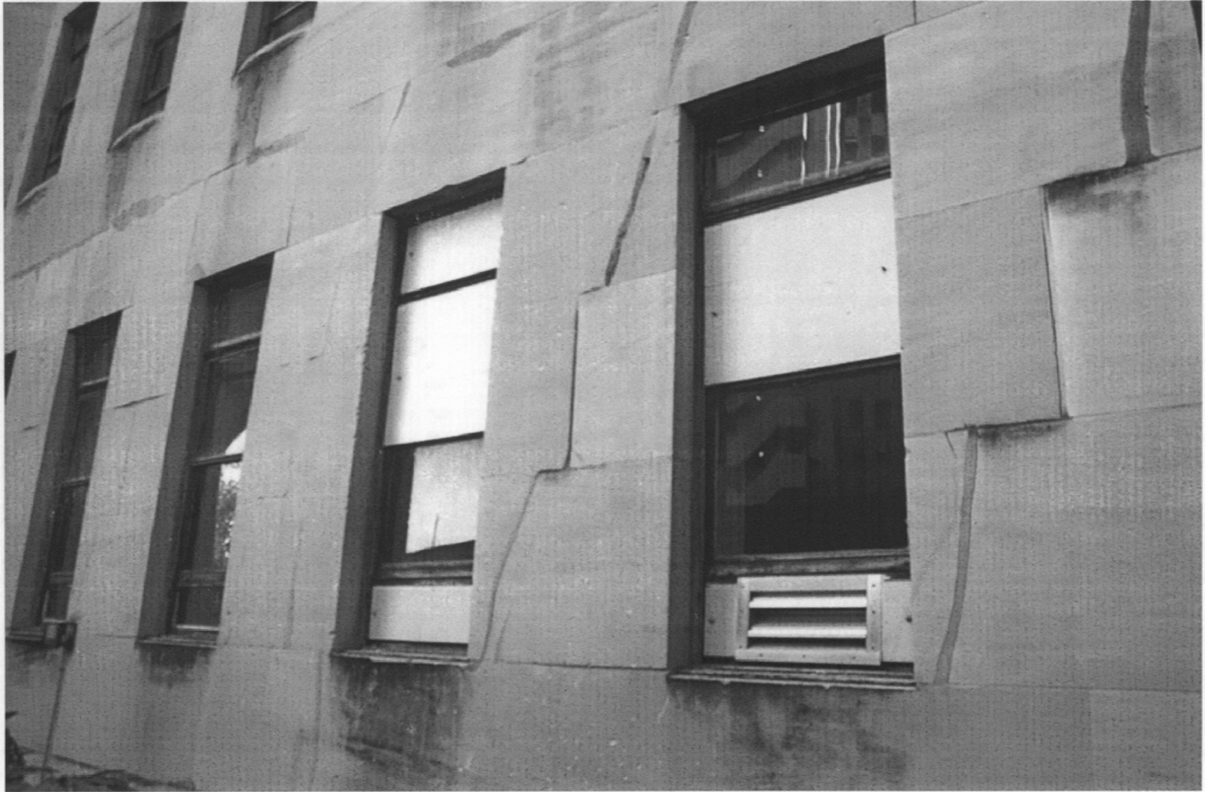
Figure 45. Charity Hospital, Cracks with repairs from settlement. Courtyard (Earth Search, Inc., July 2009).
