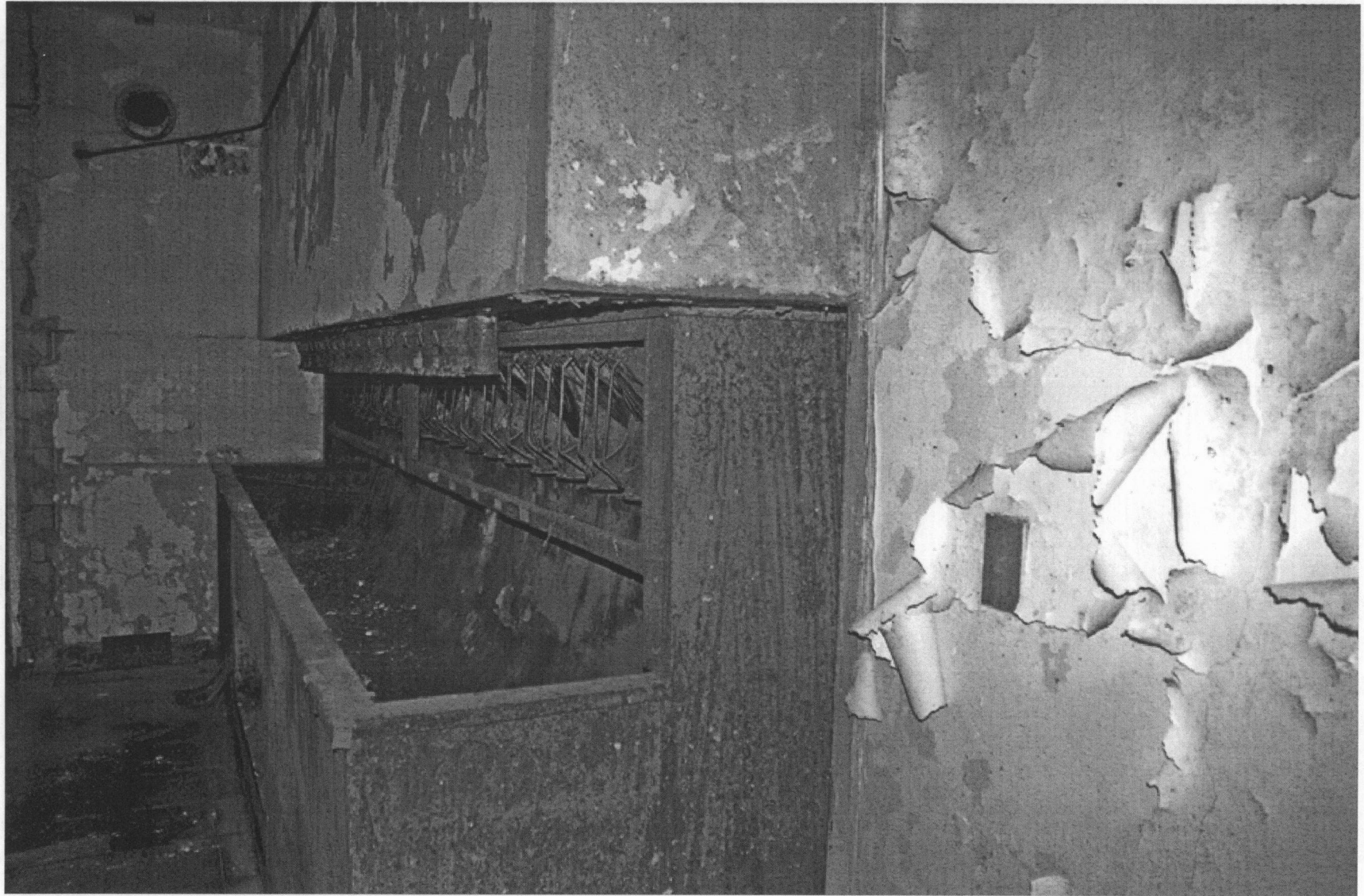
Figure 62. Charity Hospital, Pneumatic tube system central station in the basement (Robert Tucher, photographer, July 2009).
