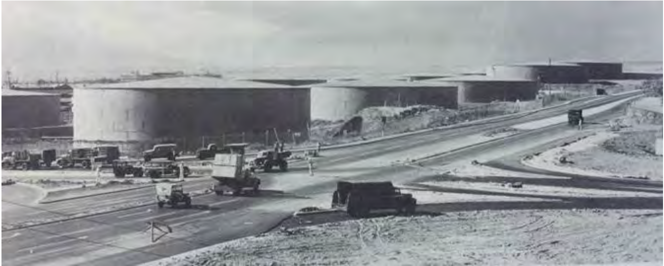
Figure 7-9. Photograph looking northwest, showing the Makalapa Gate intersection under construction, ca. 1946, with fuel tanks along Kamehameha Highway in view, and the east entry gate to Pearl Harbor on the left. Source: U.S. Department of the Navy, Bureau of Yards and Docks, Building the Navy's Bases in World War II: History of the Bureau of Yards and Docks and the Civil Engineer Corps , Vols. I & II (Washington, D.C.: United States Government Printing Office, 1947); copy on file at the archives of NAVFAC Hawai'i, Joint Base Pearl Harbor-Hickam, Honolulu, Hawai'i.
