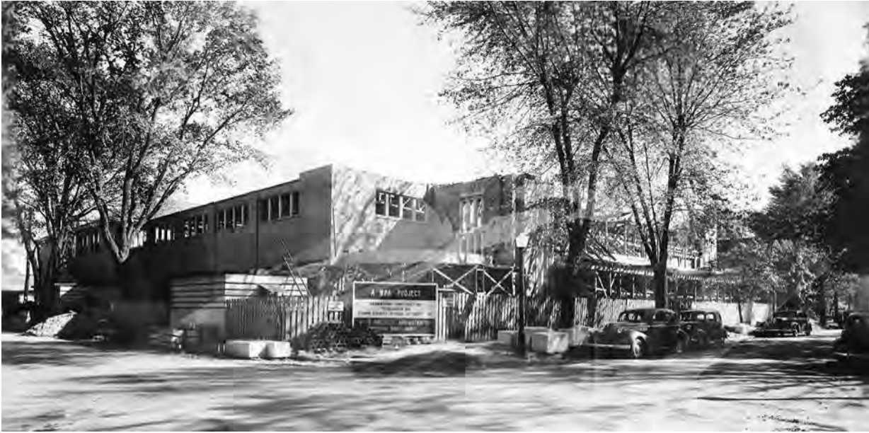
Figure 24. Paris High School Gymnasium under construction, ca. 1942. (Top: Exterior, NW corner. Bottom: Interior arena.) Source: Edgar County Historical Society.
