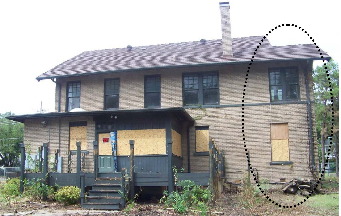
Figure 7 - Saigling House rear elevation during the recent renovation, showing the rear elevation and southeast wing (dashed area enlarged on Figure 8). There is no vertical joint or evidence of brick having been 'toothed-in' at a later date, indicating that the southeast wing is original to the house (Sept. 20, 2015).
