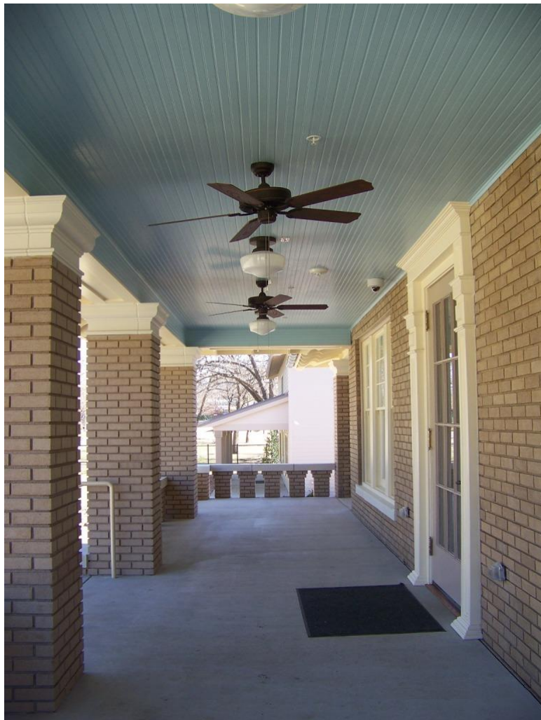
Photo 9 - View of the reconstructed front porch after renovation. Camera facing east. (February 22, 2017)
