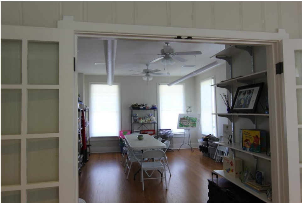
Photo 17 - Interior view of second floor southwest classroom after renovation, viewed from northwest classroom, showing open French doors salvaged from the first floor. Camera facing south. (April 6, 2017)
