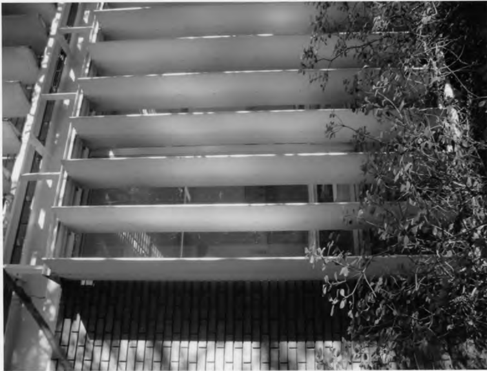
R09. Structural Science Building (Lee Hall / Lowry Hall) Clemson University Pickens County, S.C.
