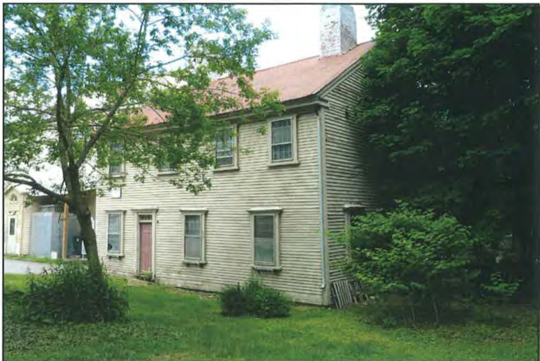
Photo 4: View northeast at west and south elevations of Dummer House. SCC, June 2017.
