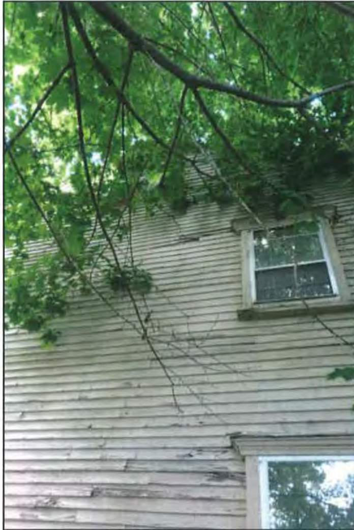
Photo 6: Detail view of south elevation of Dummer House showing overgrown tree growth impacting house. SCC, June 2017.
