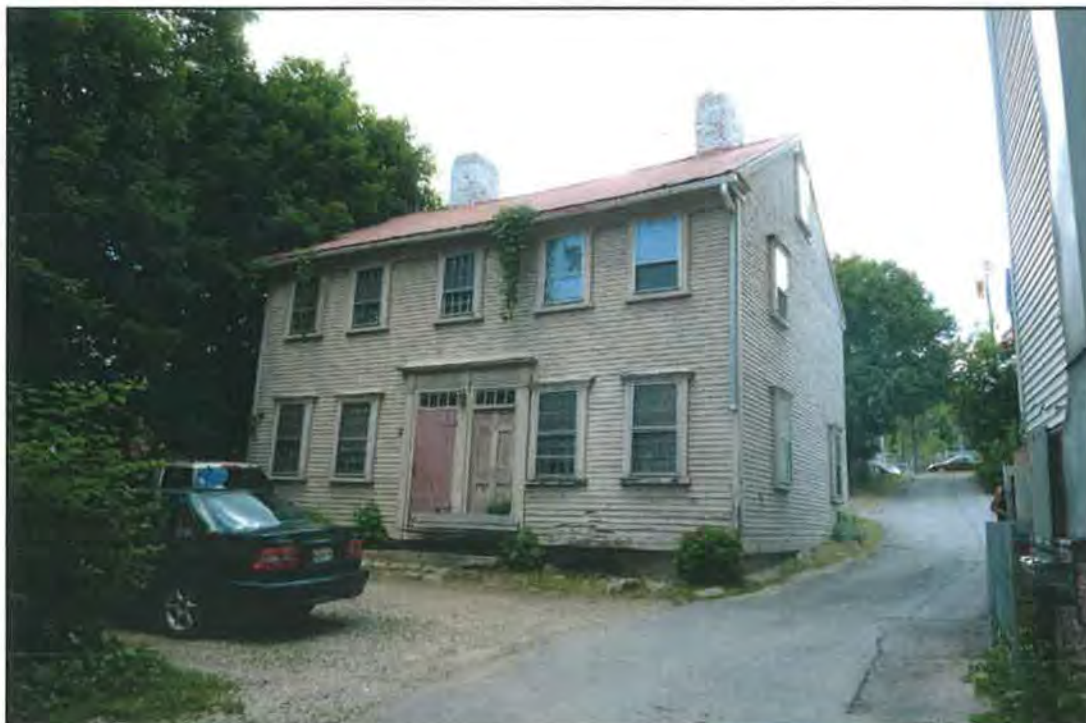
Photo 2: View southwest at east and north elevations of Dummer House from Dummer Lane. Note plant growth in eaves. Sutherland Conservation & Consulting (SCC), June 2017.
