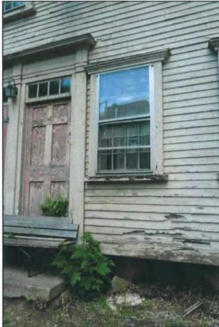
Photo 5: Detail of east elevation of Dummer House showing typical deterioration of foundation, siding and trim. SCC, June 2017.
