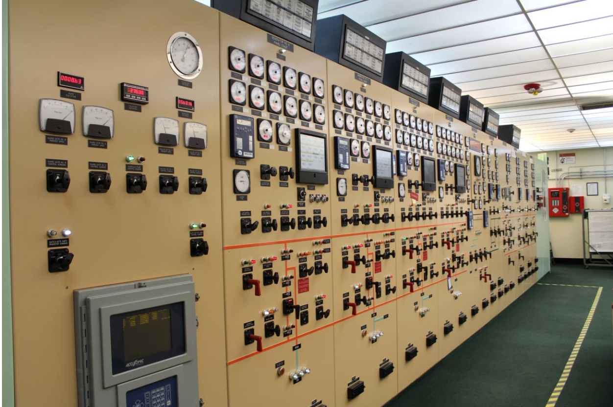
Photo 21 of 30. Interior of powerplant, original control panel. View to southwest.
