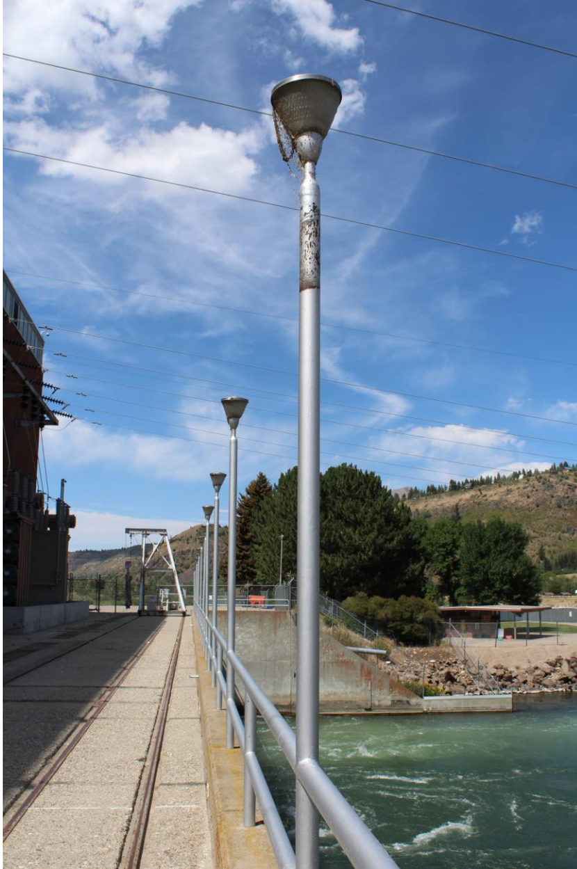
Photo 20 of 30. Powerplant transformer deck, detail of lighting. View to north.
