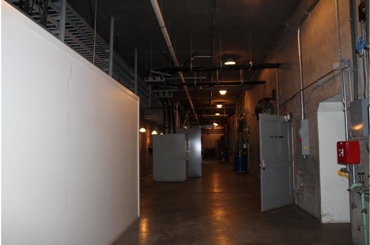
Photo 24 of 30. Interior of powerplant, lower floor two. View to south.
