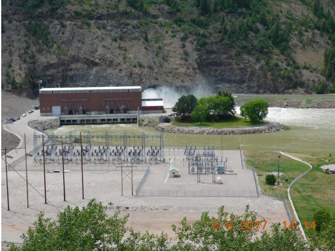
Photo 30 of 30. Vista Park on Right, Switchyard in Foreground Powerhouse to the Left. View West.
