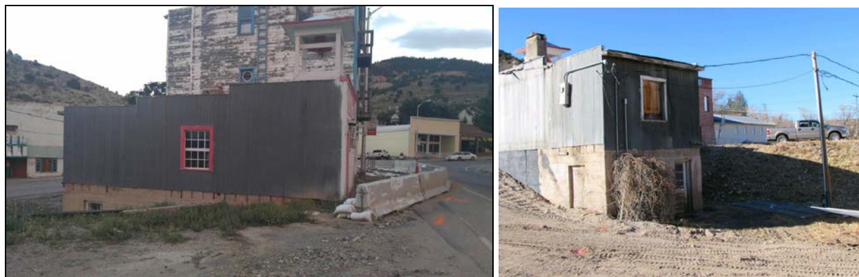
Photographs 2 and 3 – Left (2): North elevation, showing foundation and basement level, and first floor fenestration (NVSHPO, 8-11-2017); Right (3): Rear (east) elevation and southeast corner, looking northwest (Matt Elmer, December 6, 2017).
