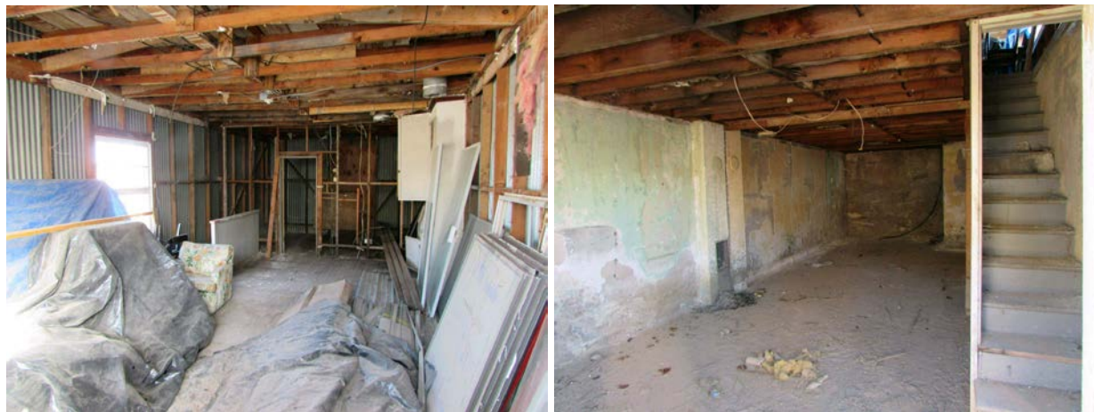
Photographs 4 and 5 – Left (4): Interior upper floor, looking east toward rear of building. Note the knee wall on the left, and tongue-and-groove flooring at center; Right (5): Lower floor, looking southwest from bottom of staircase, showing stove area (both Matt Elmer, December 6, 2017).
