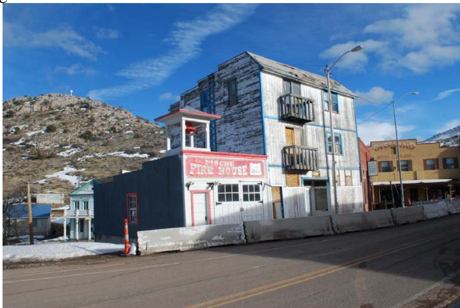
Photograph 1 – Pioche Firehouse (left), west façade facing Lacour Street, looking southeast. The two buildings to the south (photo right) of the Firehouse were demolished in the winter of 2017 due to structural damage (NVSHPO, February 8, 2017).
