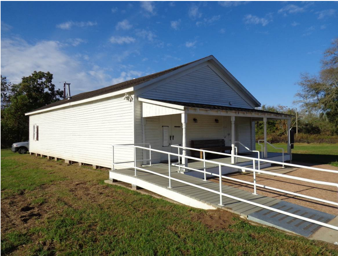
TX_Austin County_San Felipe de Austin_0005 J.J. Josey Store, east and north elevations, view southwest
