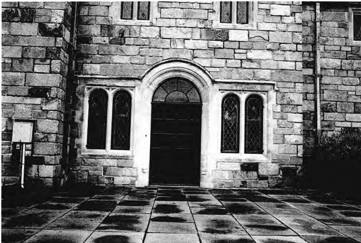
Photograph 5. Manor House, southern elevation, showing and arched doorway, flanked by paired arched casement windows, view north.
