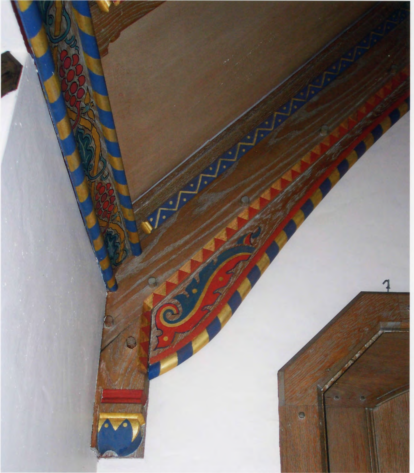
Photo # 19 Gallaher Estate-Cranbury Park, Norwalk, Fairfield County, CT Manor House, bedroom ceiling over porte-cochere showing detail, second floor, view southeast.
