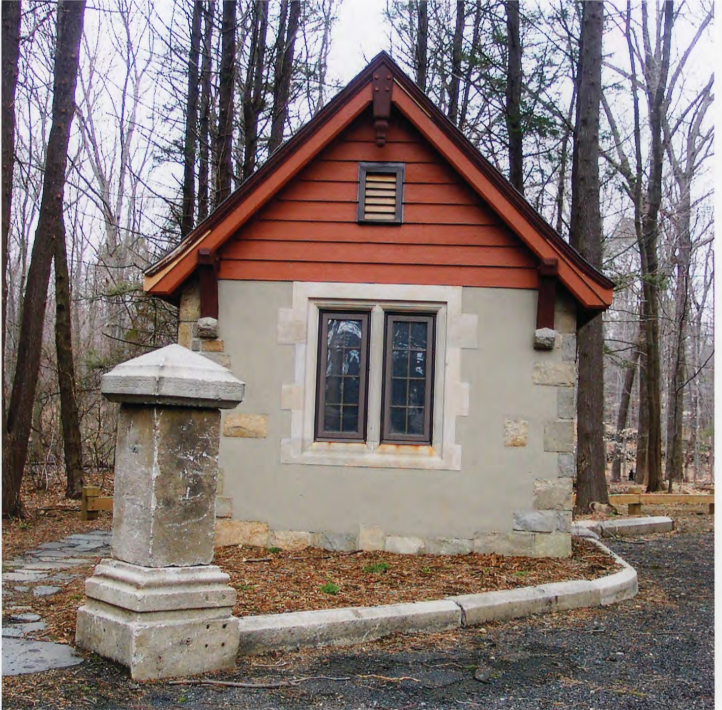
Photo # 29 Gallaher Estate-Cranbury Park, Norwalk, Fairfield County, CT Pump house, south elevation, view north.
