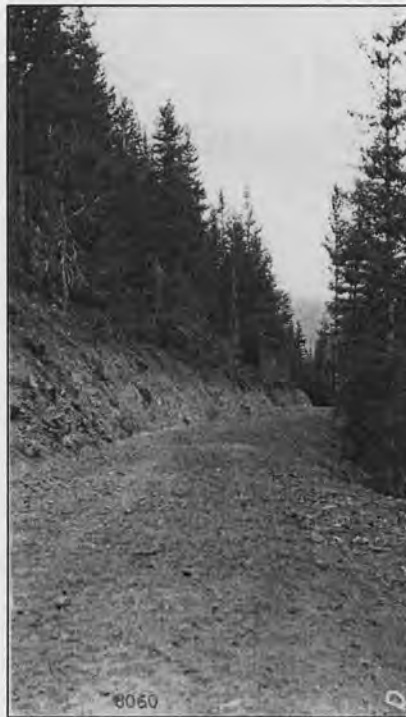
Construction on the Deadhorse Grade section in the early 1920s; view to the west (USBPR Records).
