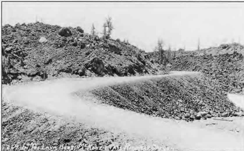
Example of cut and fill at the west entry to the lava fields in the early 1920s. (Photograph, Collection of David Sell)
