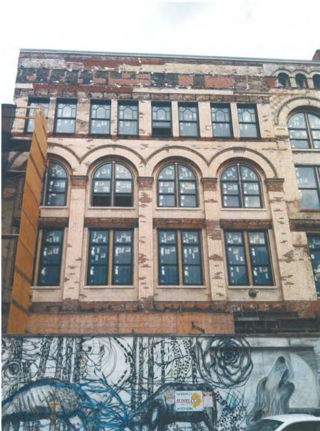
Sterchi Bros. Furniture built c. 1898 (photo: Whitney Manahan) 412 South Gay St. Non-contributing building undergoing renovation
