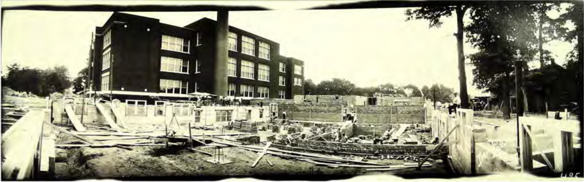
H-3 DHS Auditorium Under Construction, West Side, 1928 Courtesy of the Defiance Public Library - The Edward Bronson Collection
