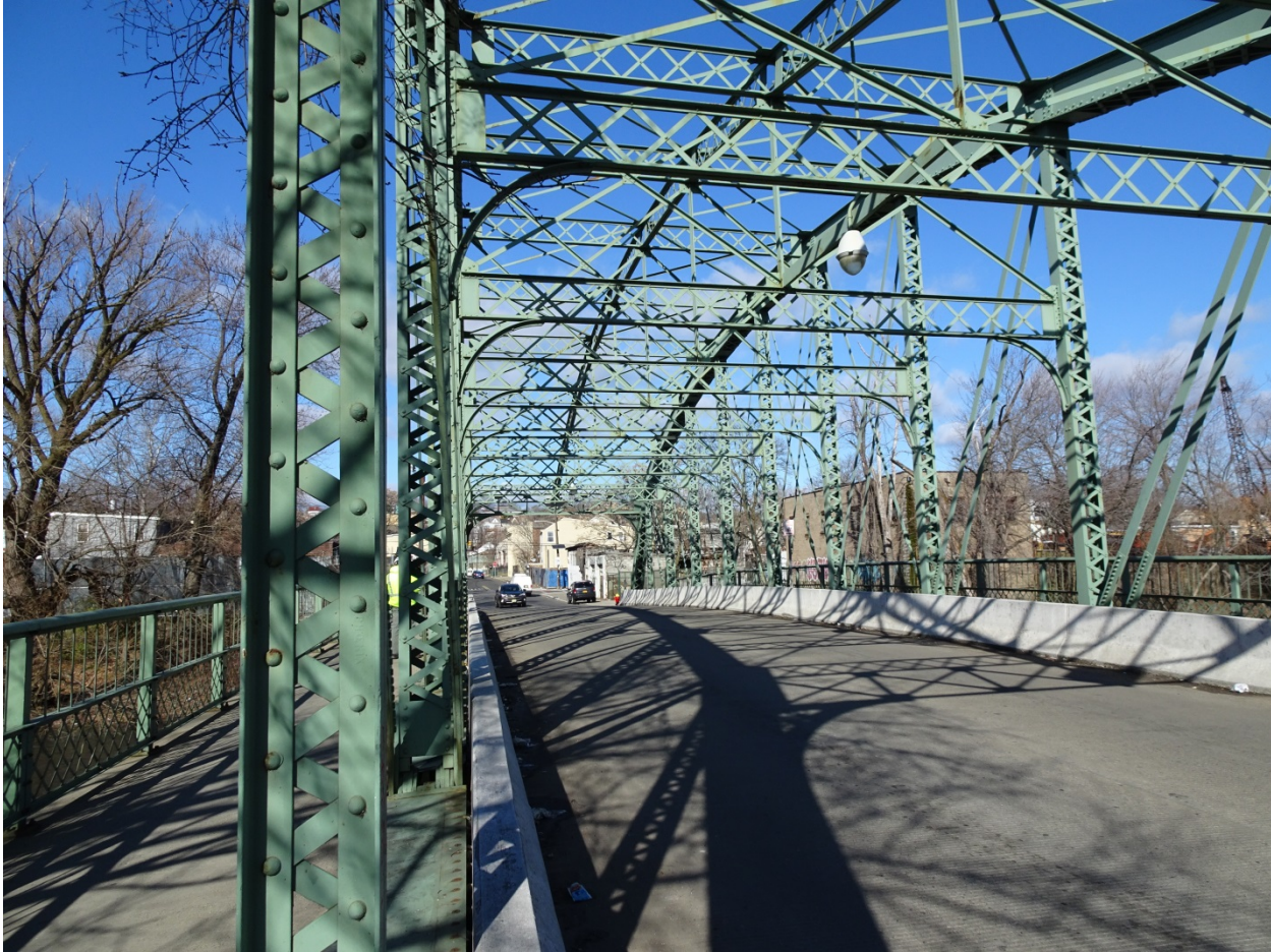
Photograph 12. View of the deck showing alterations such as a new decking and concrete Jersey barriers, view northwest.
