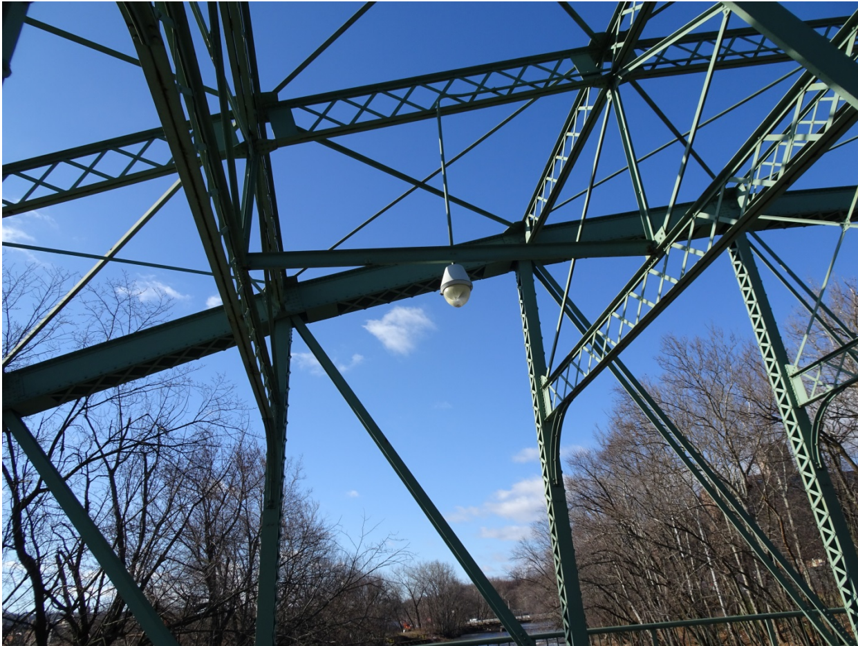
Photograph 7. Truss detail, showing the polygonal top chord, stepped-length verticals, and diagonals in panels, view west.
