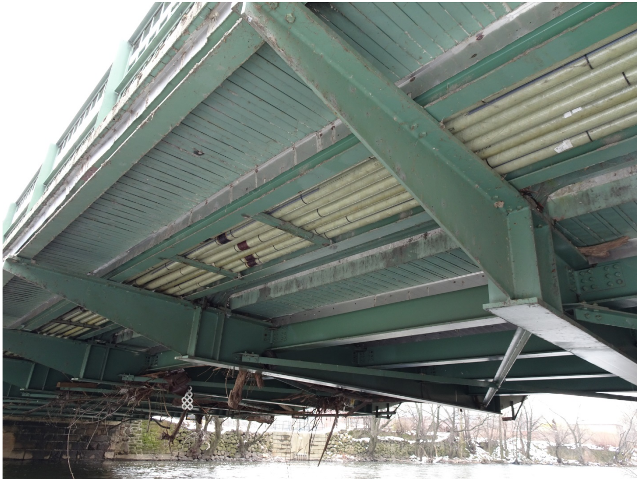
Photograph 13. View of the rehabbed floorbeam and stringer system and the debris caught in the substructure of the bridge, view south.
