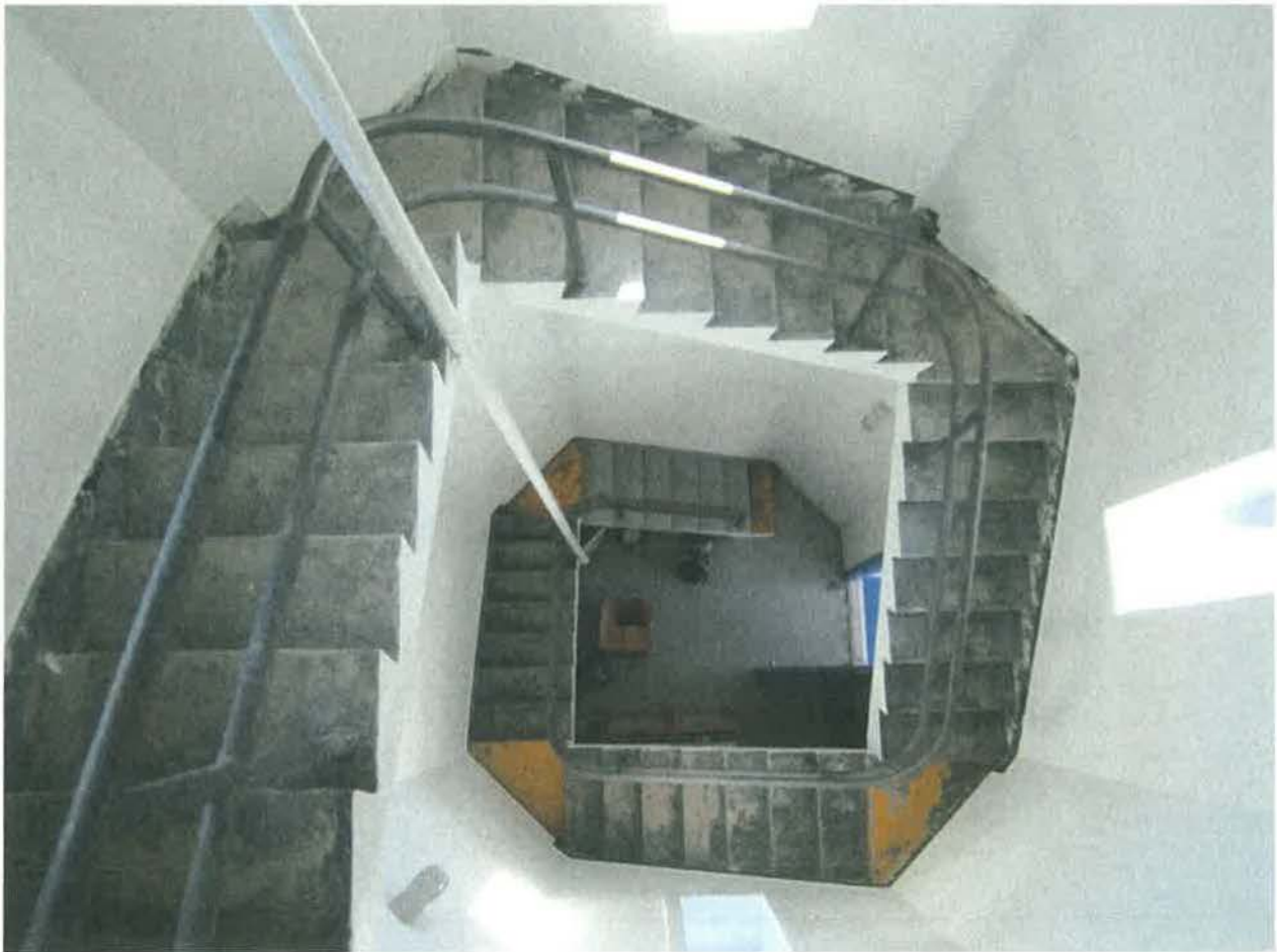
Photo # 4. Light tower interior looking downward from service room, camera facing down towards southeast.
