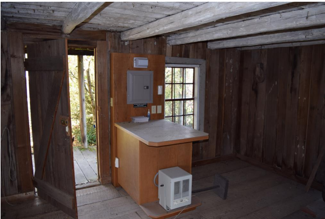
9 of 15. Interior looking at northwest corner showing entry and registration desk with electrical panel and heater.
