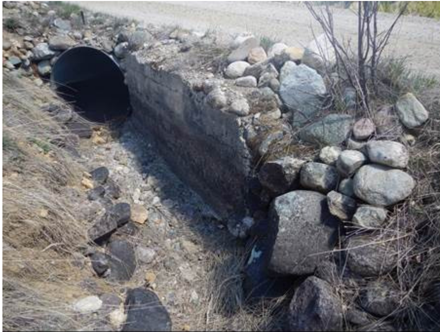
Photograph 16. MT_CarbonCounty_RockCreekRangerStationHD_0016. Maryott Ditch, steel pipe culvert and concrete wall to the west of the District's access road, facing northeast (Source: Logan Simpson, 2015).
