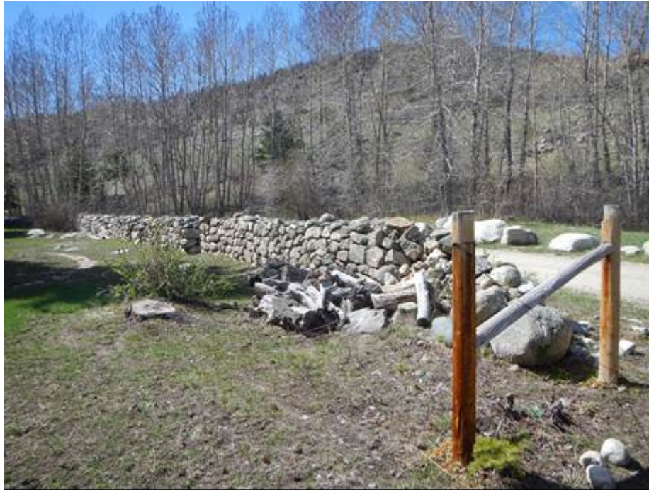
Photograph 13. MT_CarbonCounty_RockCreekRangerStationHD_0013. Stacked stone wall to the north of the main cabin (Building #1010), facing southwest (Source: Logan Simpson, 2015).
