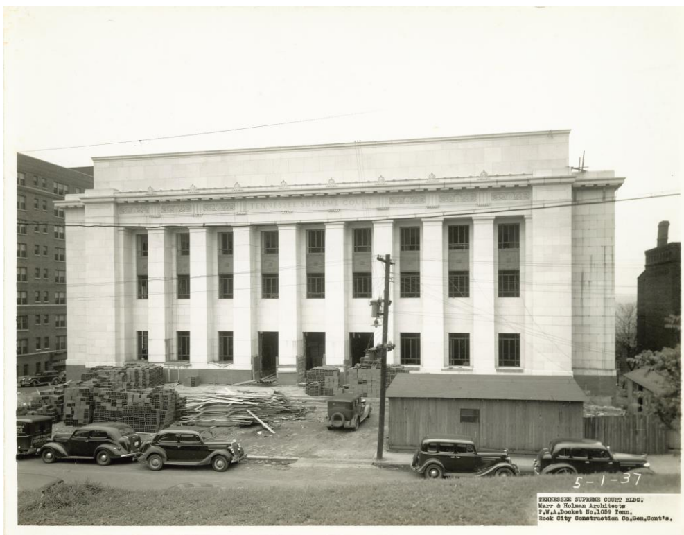
Figure 18. Construction progress May 1, 1937. (Courtesy of Rock City Construction and the Tennessee Supreme Court)
