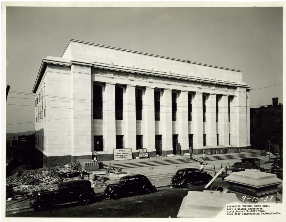
Figure 22. Construction progress September 15, 1937. (Courtesy of Rock City Construction and the Tennessee Supreme Court)
