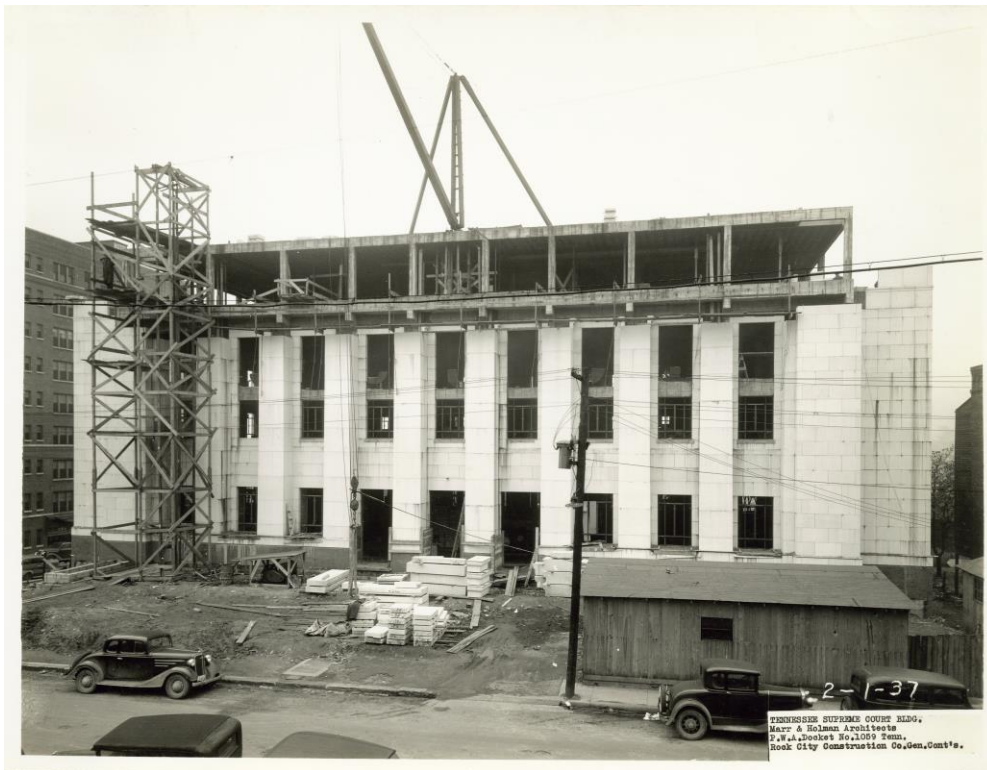
Figure 15. Construction progress February 1, 1937. (Courtesy of Rock City Construction and the Tennessee Supreme Court)
