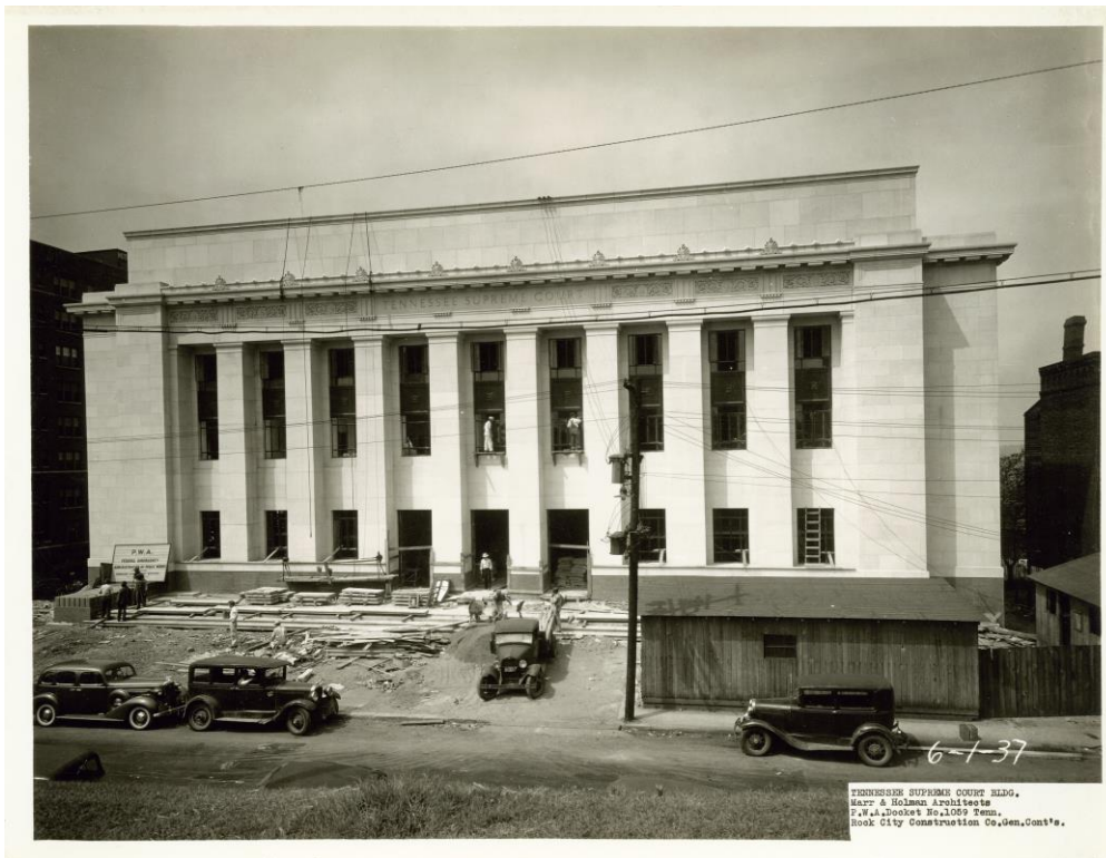
Figure 19. Construction progress June 1, 1937. (Courtesy of Rock City Construction and the Tennessee Supreme Court)
