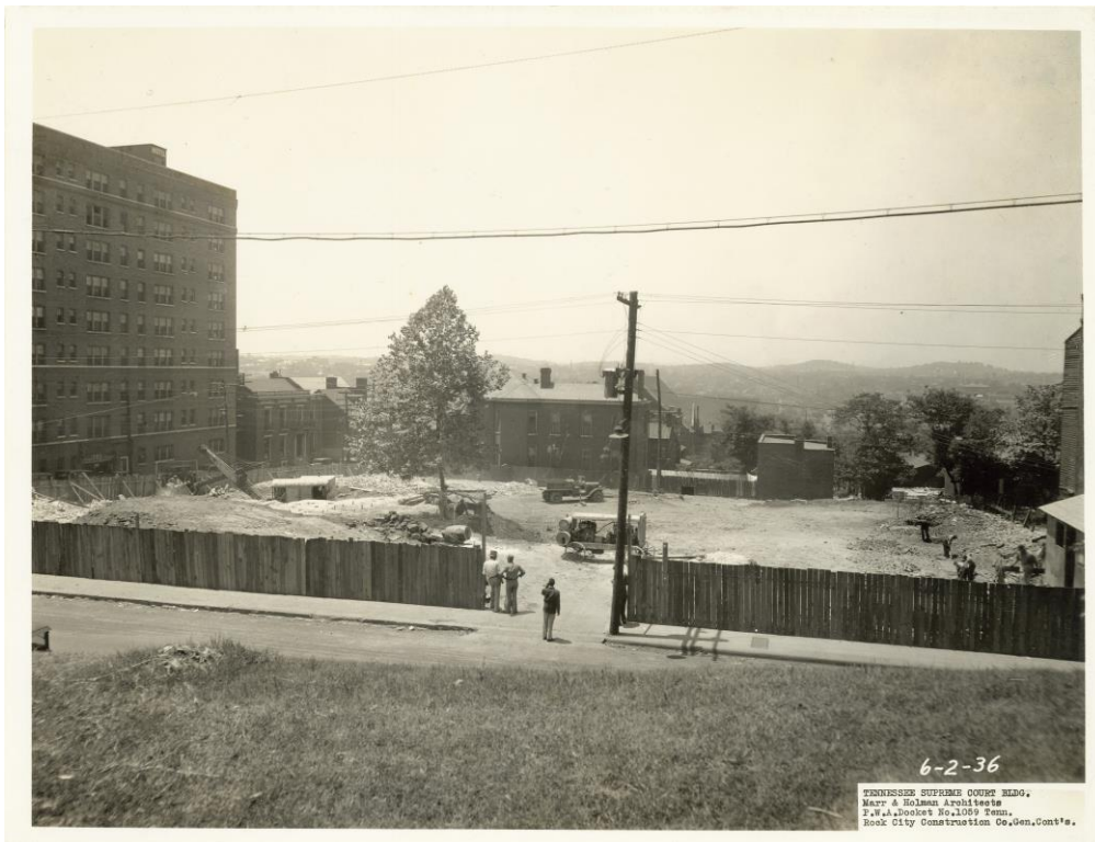
Figure 7. Construction progress June 2, 1936. (Courtesy of Rock City Construction and the Tennessee Supreme Court)
