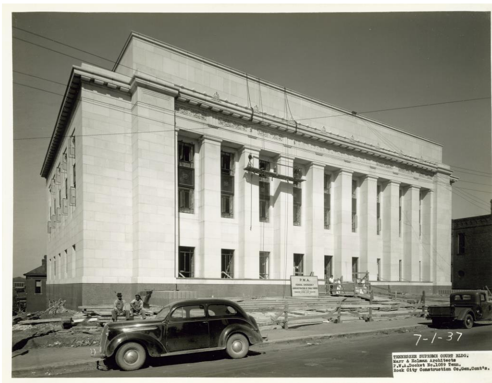
Figure 20. Construction progress July 1, 1937. (Courtesy of Rock City Construction and the Tennessee Supreme Court)
