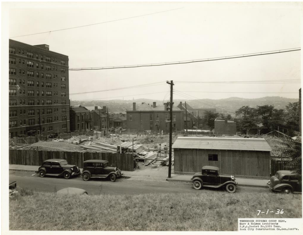
Figure 8. Construction progress July 1, 1936. (Courtesy of Rock City Construction and the Tennessee Supreme Court)
