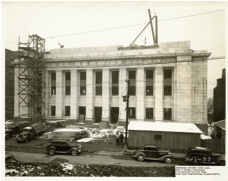
Figure 16. Construction progress March 1, 1937. (Courtesy of Rock City Construction and the Tennessee Supreme Court)
