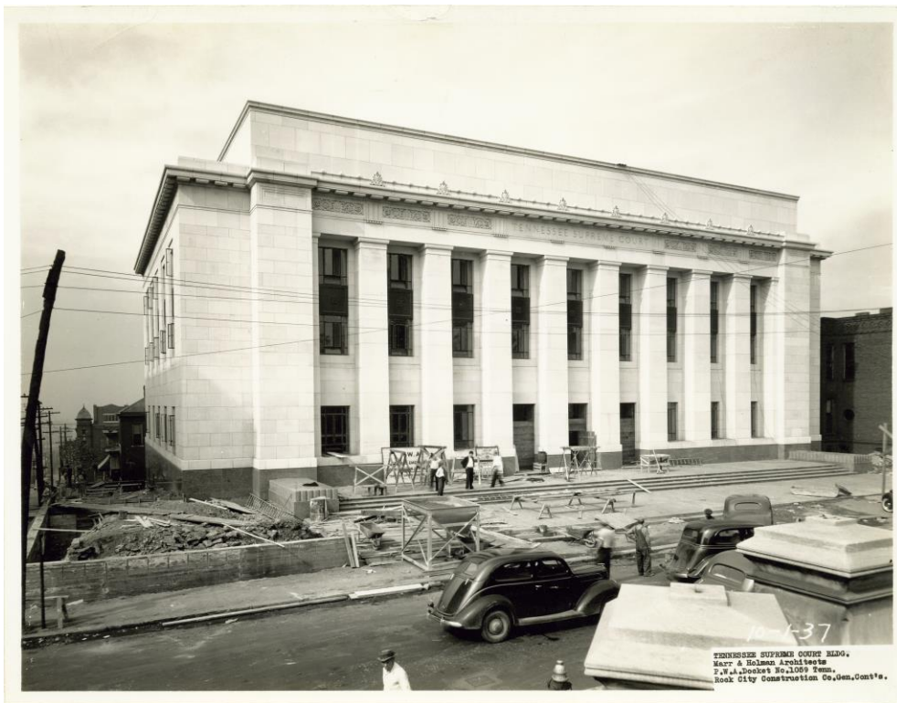
Figure 23. Construction progress October 1, 1937. (Courtesy of Rock City Construction and the Tennessee Supreme Court)
