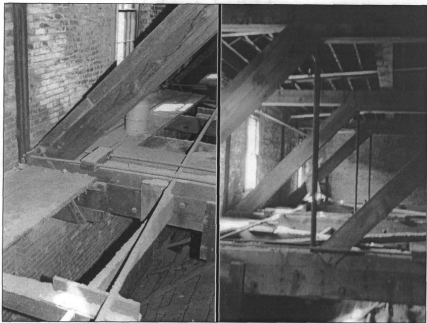
Figures 29 and 30: Left, attic truss juncture with west sidewall, note the angled auditorium ceiling below Right, three attic trusses, note mortise cuts and steel compression bars, view north (photos by James Jacobsen, August 2001)
