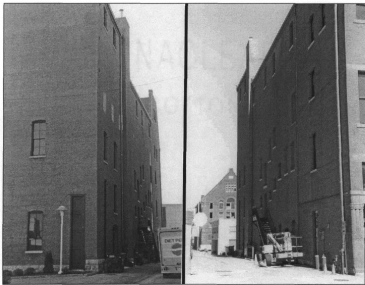
Figure 6 and 7: Left, west side wall, view to south, Right, same, view to north (photos by James Jacobsen, August 2001)
