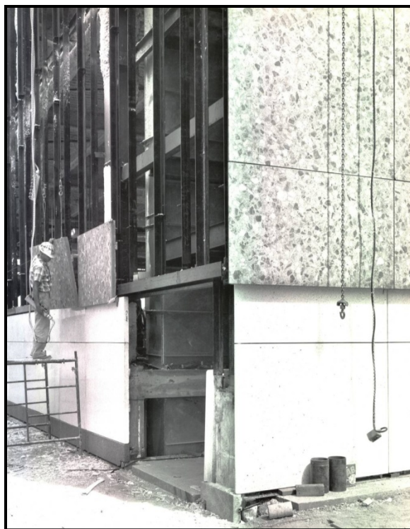
H8. August 1, 1963, photograph of pre-cast concrete southeast corner of the U.S. Courthouse.
