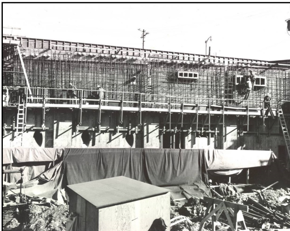
H5. December 6, 1962, photograph of construction progress showing the installation of reinforcing steel.
