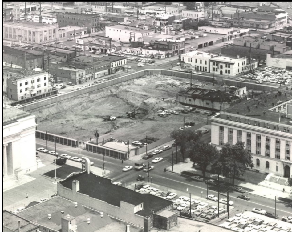
H3. June 1, 1962, photograph of the excavation from the southeast corner, facing northwest.
