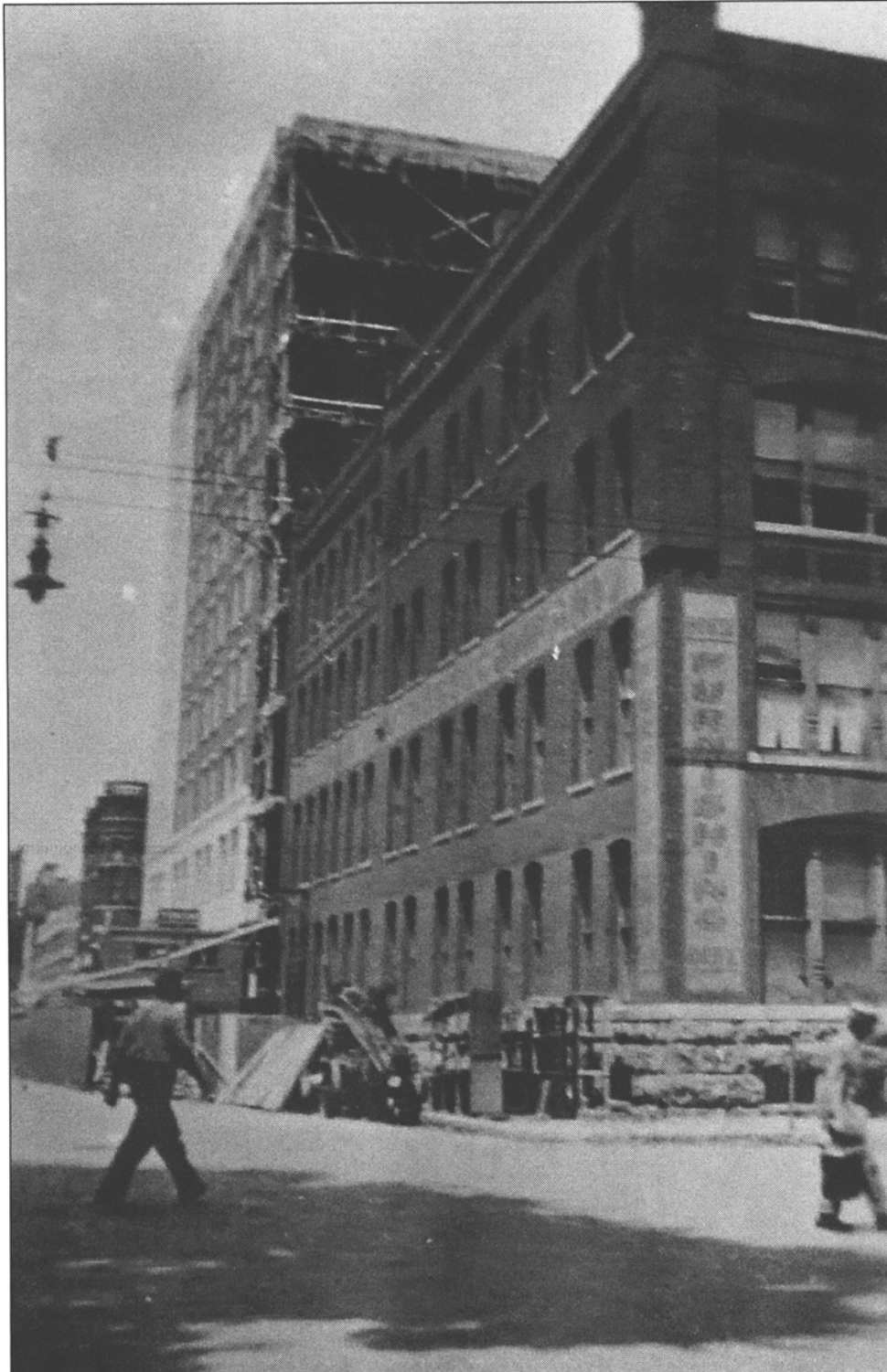
Figure 16: Roshek building construction photo, view north, mid-1930 (Loras College, Center for Dubuque History, Photo NGL-1672)
