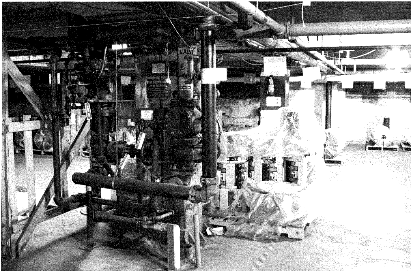
Photo 22 of 23: Basement: sprinkler equipment. View to SE.
