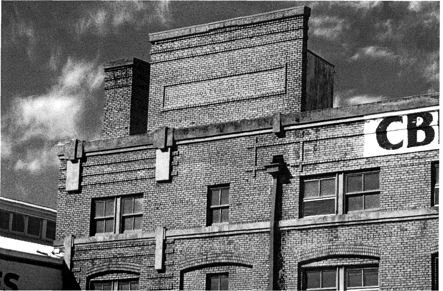
Photo 9 of 23: Southwest façade: parapet, chimney, and elevator overrun detail. View to NE.
