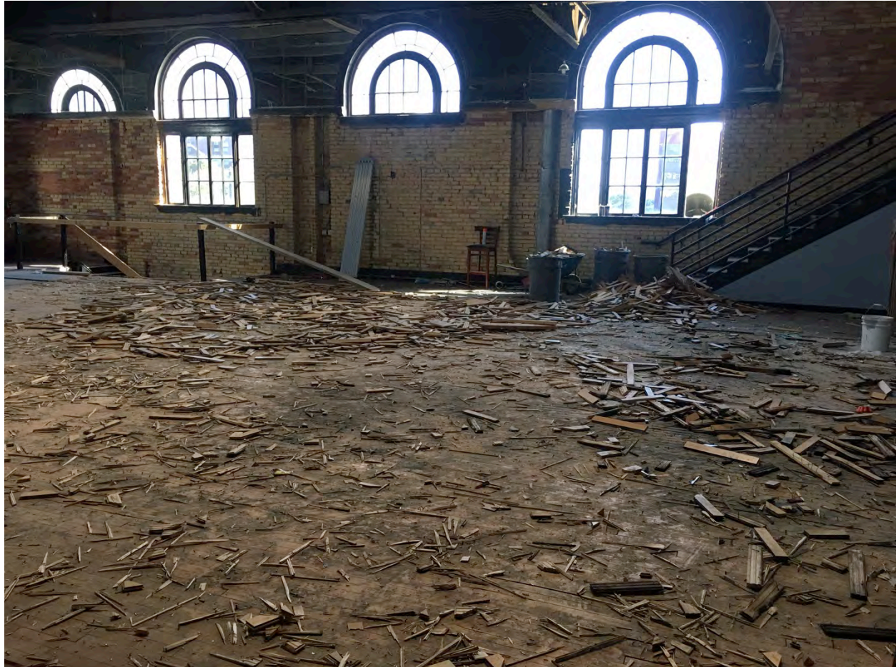
Pre-rehabilitation Photograph Figure No. 5 of 5, Second floor level, event space. Camera facing south. *Photographed in January 2018.
