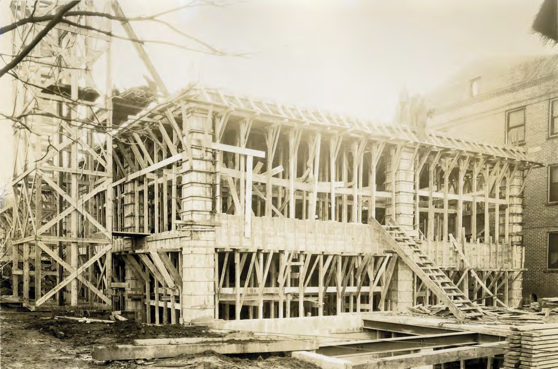
FEDERAL LAND BANK BUILDING COLUMBIA, S. C. J. C. HESLER, CONT. LAFAYE & LAFAYE, ARCH.
