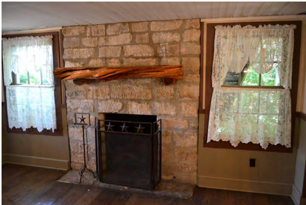
Photo 16. Current photograph (facing south) of the southeastern fireplace on the first floor of the original 1860 building. Wall finishes, fireplace details, and hardware have changed. Wooden floors, ceilings, and window and door trim likely date to the period of significance. Compare to the historic photograph in Figure 13. Source: HHM, 2016.
