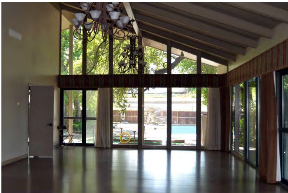
Photo 41. Current photograph (facing west) from the interior of the 1960 clubhouse building (Resource 4) facing out into the side pool area (Resource 10). The exposed wood rafter ceiling and window wall are original, but other finishes and fixtures are not. Compare with the historic photograph in Figure 20. Source: HHM, 2016.
