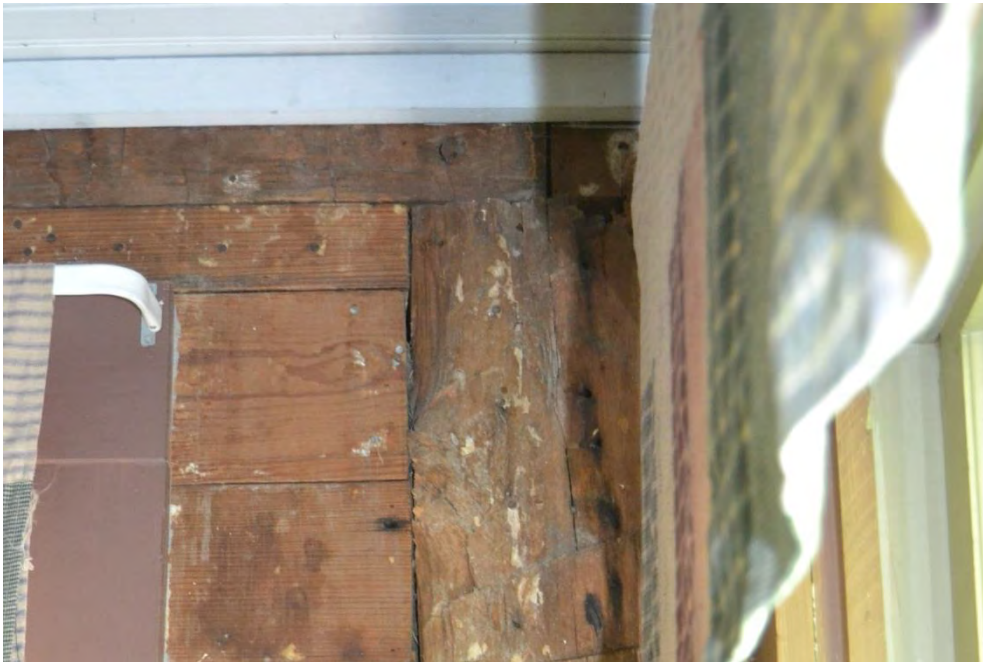
Photo 22. Current photograph (facing east) of an exposed post-and-girt structural joint in the original 1860 building, as seen at the southeast corner of the second floor. In many locations throughout the building, unhewn and rough-hewn wood structural elements are visible. Source: HHM, 2016.
