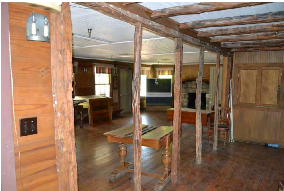
Photo 15. Current photograph (facing south) of the second floor of the original 1860 building. The roof structure is supported by a central load-bearing wall dividing the front and rear rooms. In many locations throughout the building, unhewn and rough-hewn wood structural elements are visible. Source: HHM, 2016.
