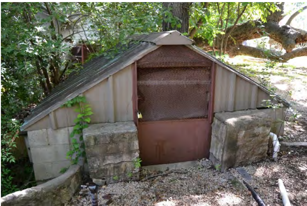
Photo 11. Current photograph (facing north) of the late 1960s or 1970s enclosure over a spring water cave. Compare to the historic photograph in Figure 16. Source: HHM, 2016.
