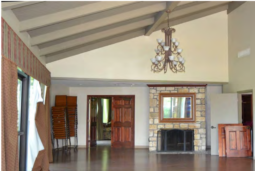
Photo 42. Current photograph (facing east) from the interior of the 1960 clubhouse building (Resource 4). The exposed wood rafter ceiling and stone fireplace are original, but other finishes and fixtures are not. Compare with the historic photograph in Figure 21. Source: HHM, 2016.
