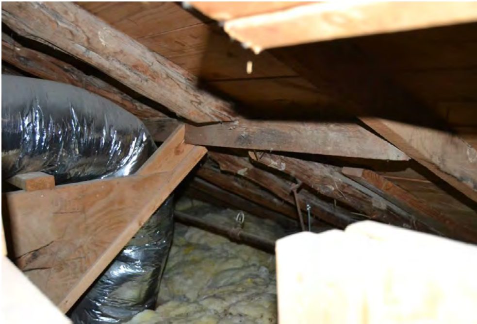
Photo 20. Current photograph (facing northeast) of the roof structure in the original 1860 building, as seen in the attic. Note that older components such as the un-hewn wood rafters have been reinforced by more recent structural members. These conditions are visible in the attic and basement. Source: HHM, 2016.
