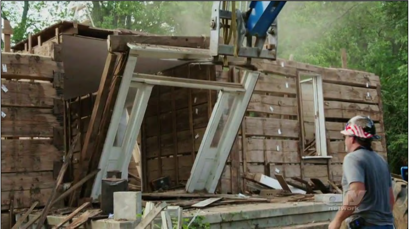
Figure 12: Screenshot of the removal of the Front Door of the Noblit-Lytle House, 2017. From “Barnwood Builders” and the DIY Network.
