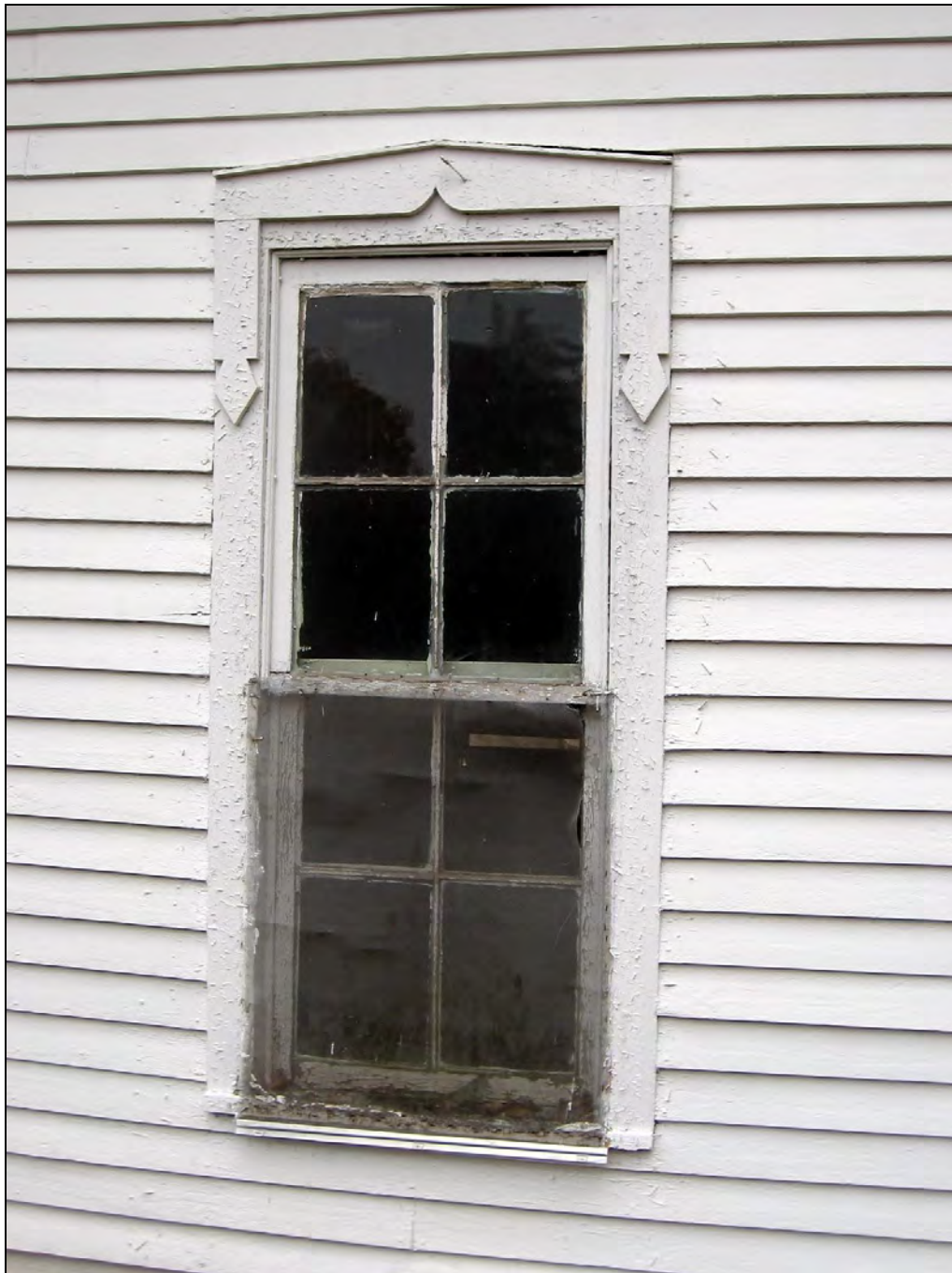
Figure 5: Noblit-Lytle House, Rear Ell Window Detail, from the Noblit-Lytle House National Register Nomination, 2008
