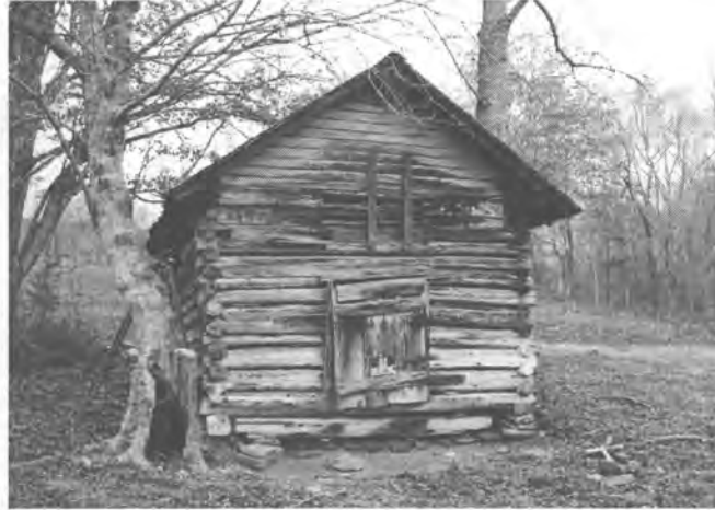
The log smokehouse was constructed in the 19 th century and retains stone chinking (R. Jones, 12/2007).
