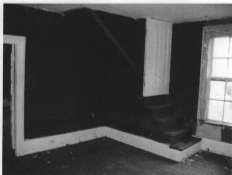
The dining room retains the enclosed corner stair that may have originally been located in the 1890s from the 1840s south parlor; its dimensions match the 1840s north parlor stair (R. Jones, 12/2007).
