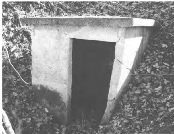
The small, concrete springhouse was built to protect a steep hillside spring around 1950; it continues to supply water to the house via a gravity-fed hose (R. Jones, 2/2008).
