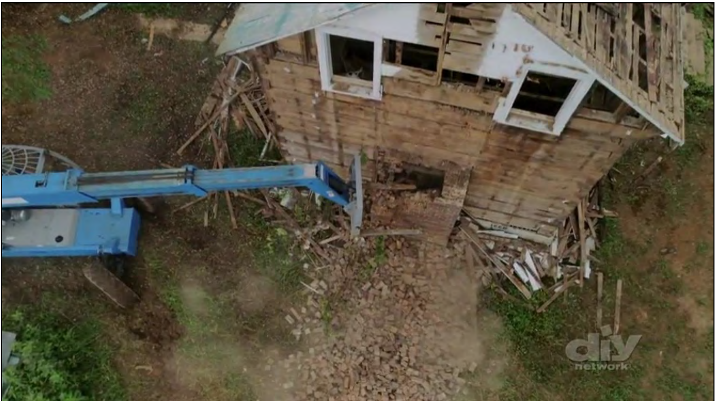
Figure 11: Screenshot of the Destruction of the Noblit-Lytle House, 2017. From “Barnwood Builders” and the DIY Network.
