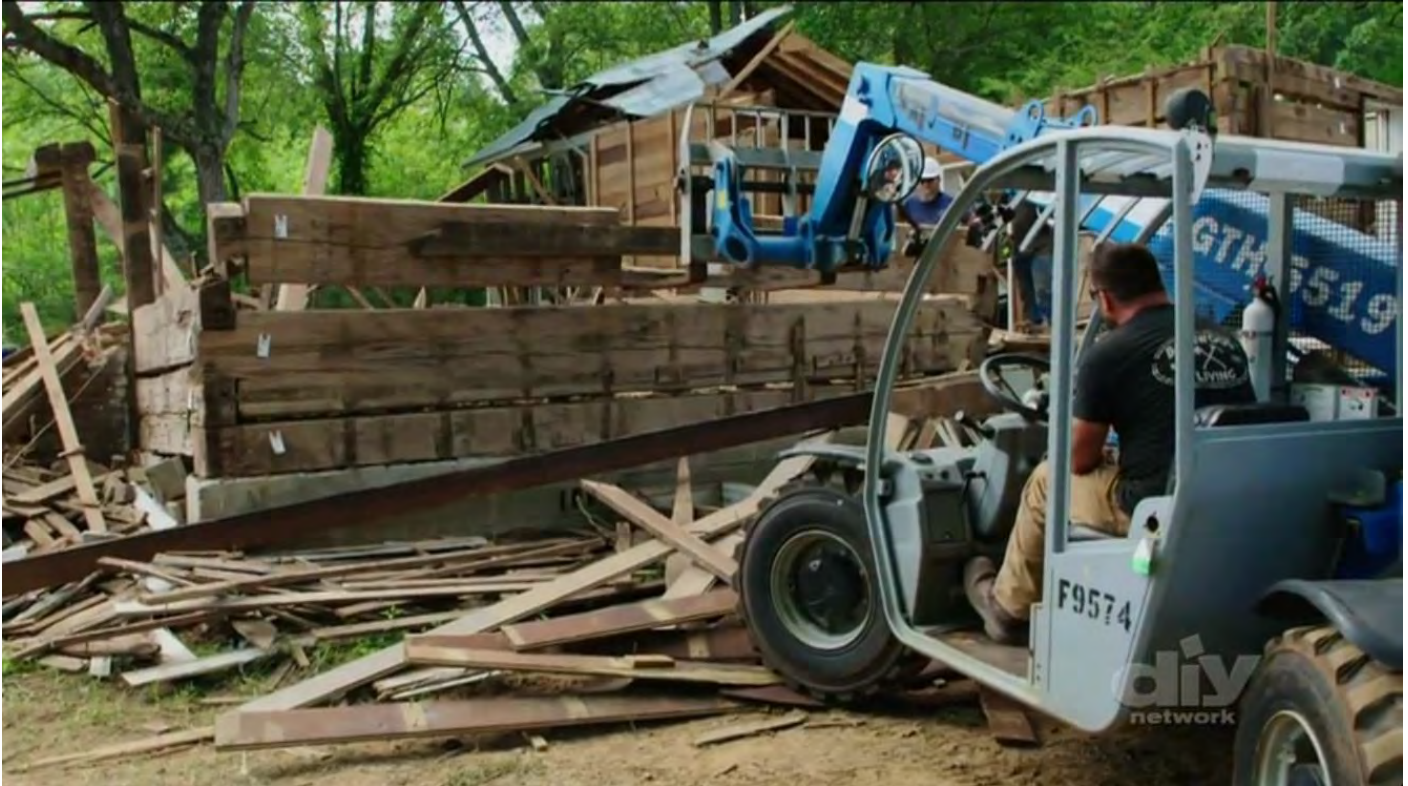
Figure 13: Screenshot of the Removal of the Logs from the Noblit-Lytle House, 2017. From “Barnwood Builders” and the DIY Network.
