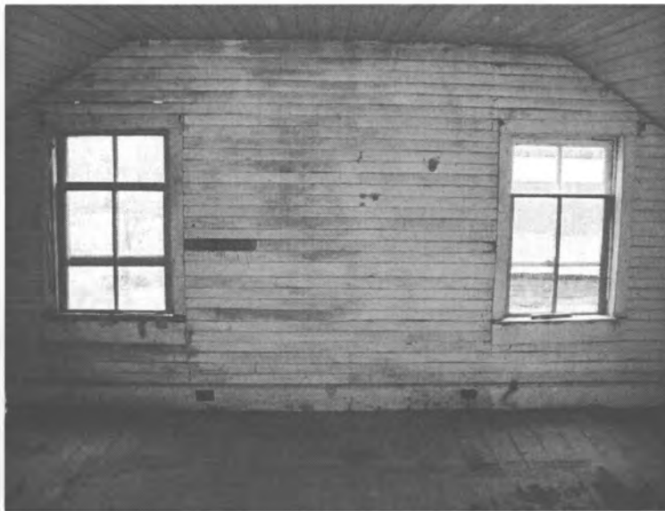
The south bedroom features beaded wallboards; the original 1840s corner stair was removed in the 1890s; the replacement floorboards are visible (right). This room was painted white. Note the "ghost" of the imported Asian floor matting dating from the early 20 th century (R. Jones, 12/2007).
