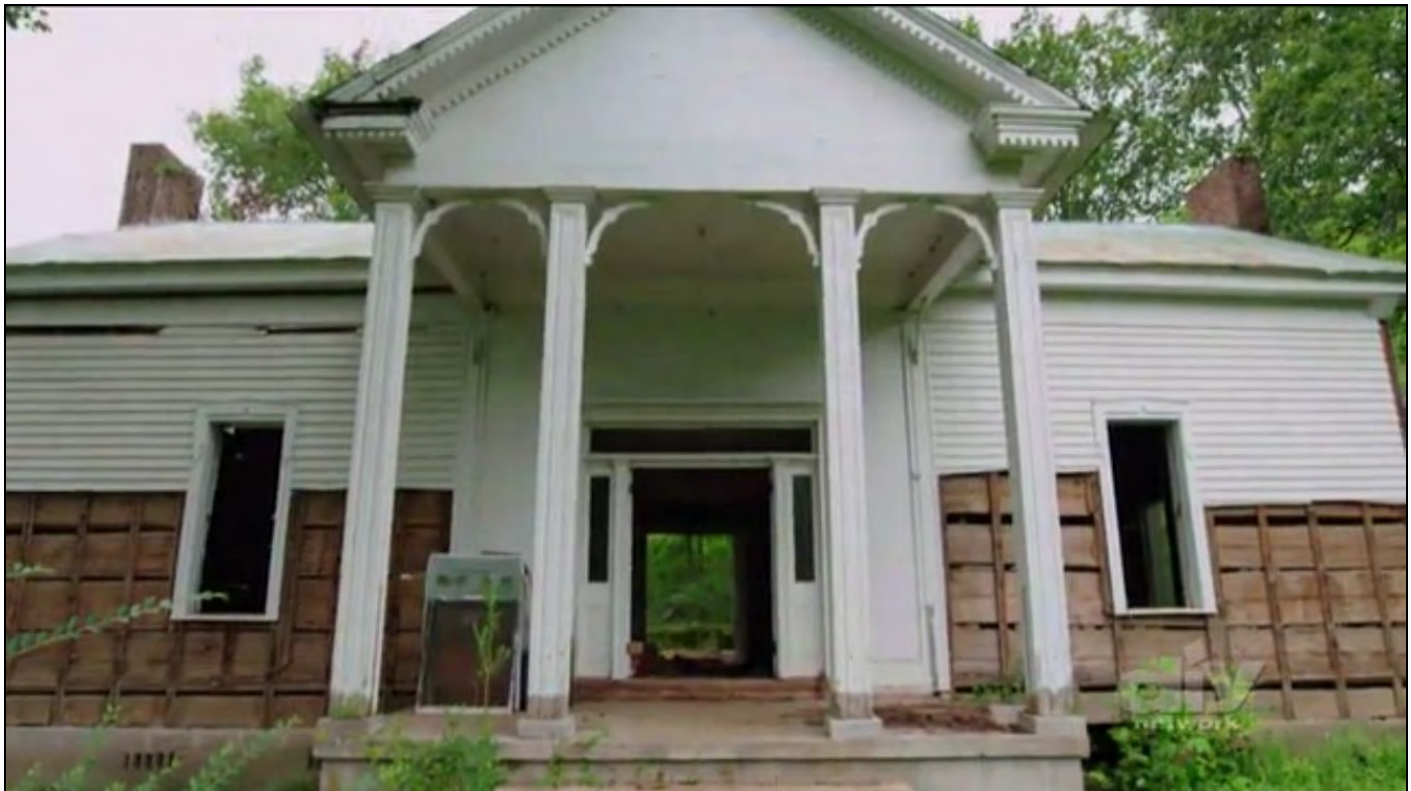
Figure 7: Screenshot showing the removal of siding on the Noblit-Lytle House, 2017. From “Barnwood Builders” and the DIY Network.
