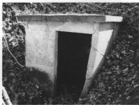
The small, concrete springhouse was built to protect a steep hillside spring around 1950; it continues to supply water to the house via a gravity-fed hose (R. Jones, 2/2008).
